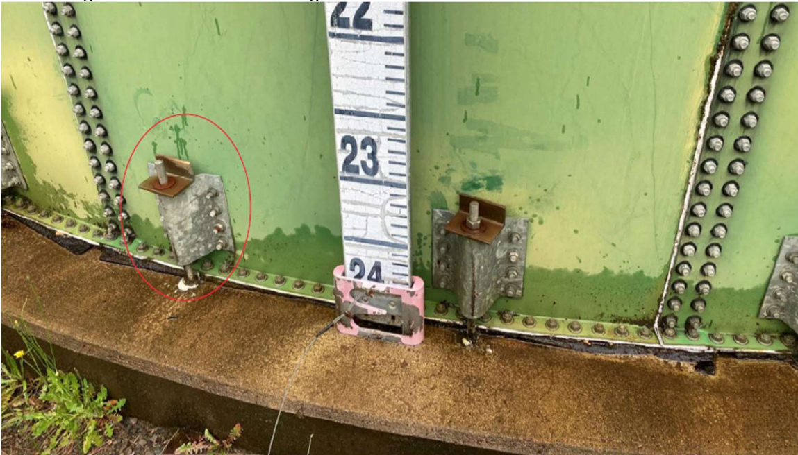
Figure 6.7 Strawberry Reservoir Anchor Bolts
