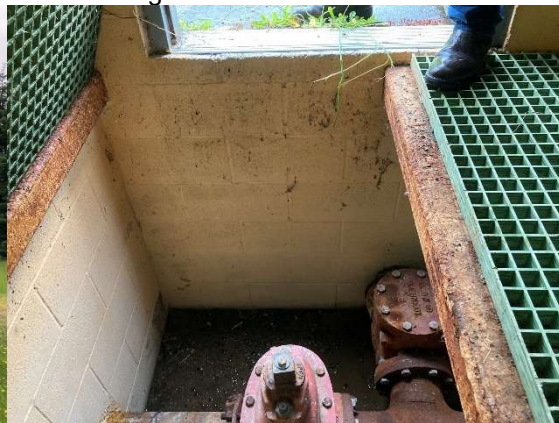
Figure 6.8.2 Strawberry Vault Corrosion
