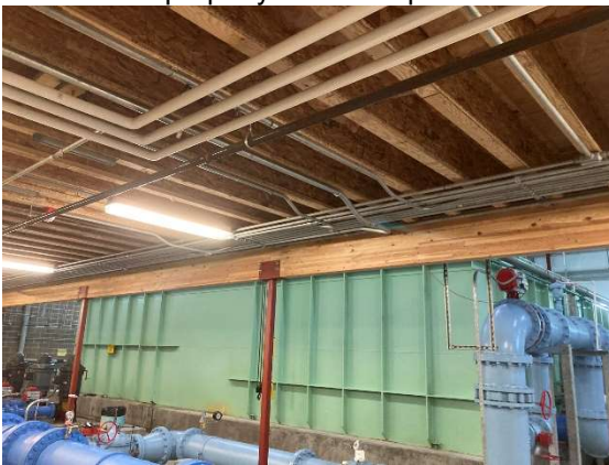
Fig 6.3.1 Open Mezzanine Lacks Redundancy
