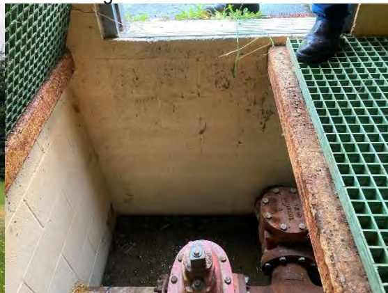
Figure 6.8.2 Strawberry Vault Corrosion
