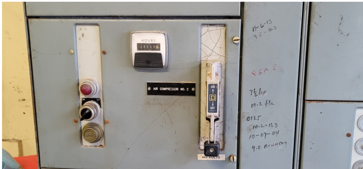
3: Solids Building - MCC Air Compressor Bucket
