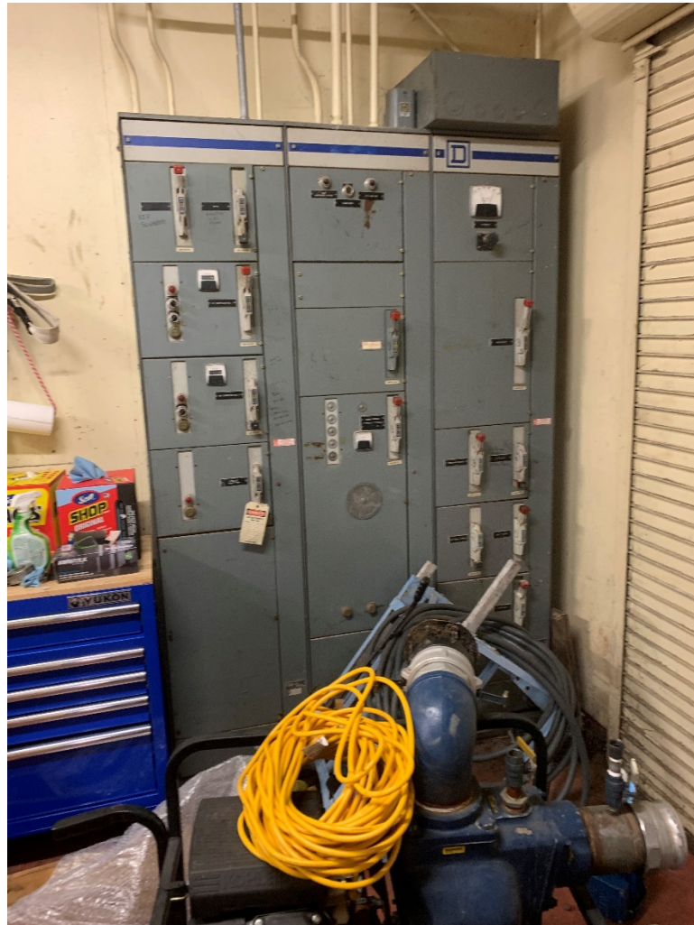
1: Solids Building - MCC Overall
