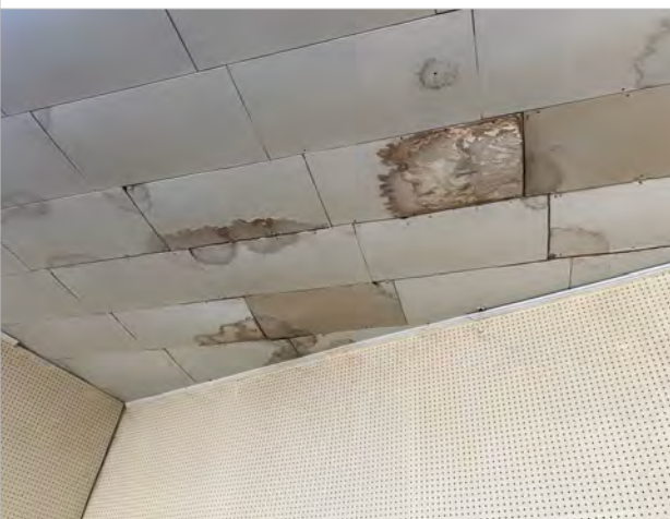
Sales Floor: Water-damaged ceiling tiles
