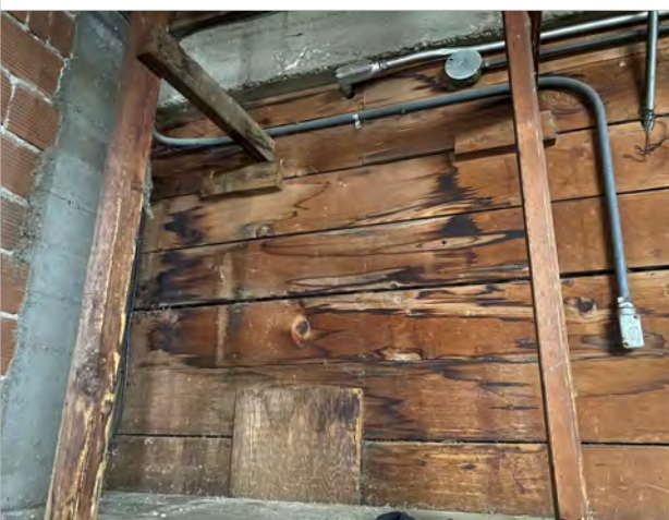
Scale Room: Water staining on wall
