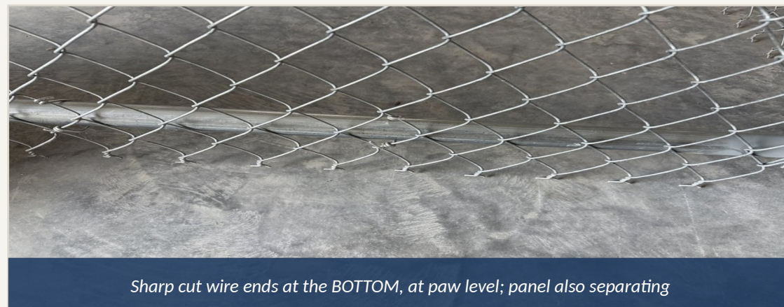
Rounded “knuckled” edge left at the TOP — the reverse of a safe install
