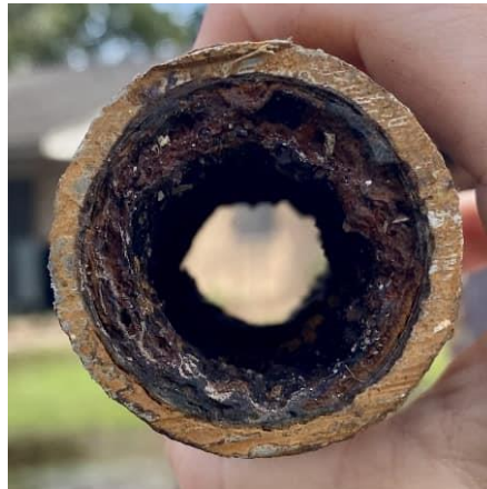
Section removed from Pecan St. waterline when staff repaired a major leak at Pecan & 4 th St. in August 2023.
