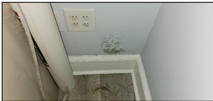
22. Visible growth on drywall near plenum
