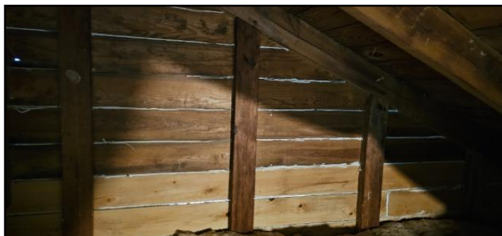
38. Gaps between wood siding
