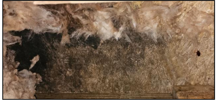
73. Visible mold growth
