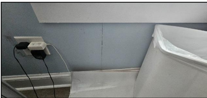
9. Visible growth at baseboard
