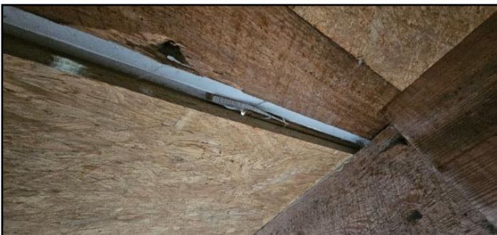
58. Exposed drywall in crawl
