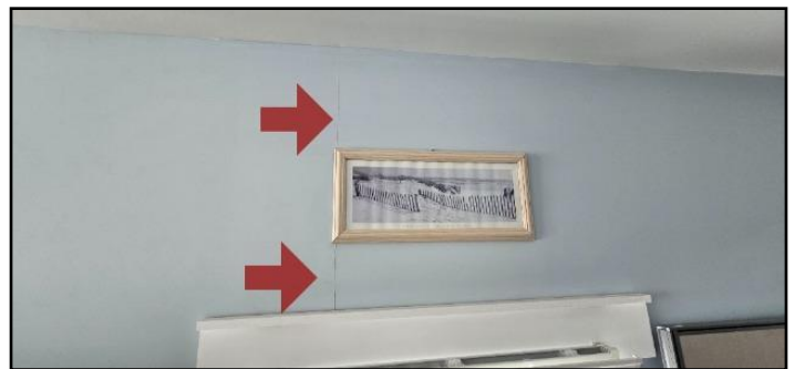
10. Crack in drywall
