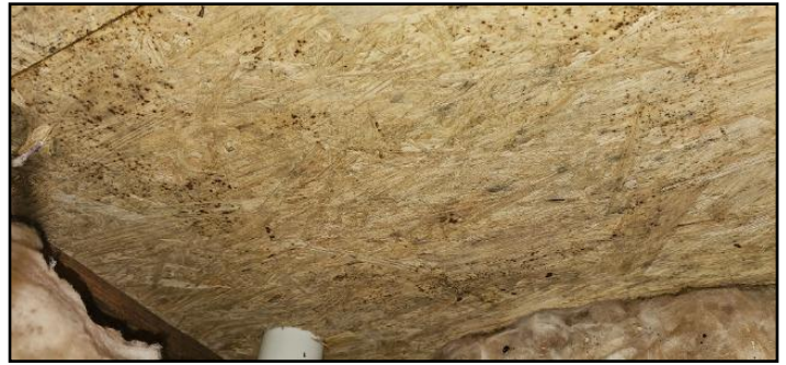
81. Visible growth on subfloor
