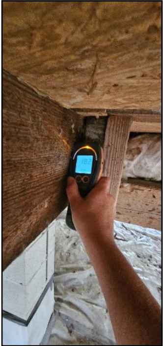
62. Wet drywall exposed in crawlspace
