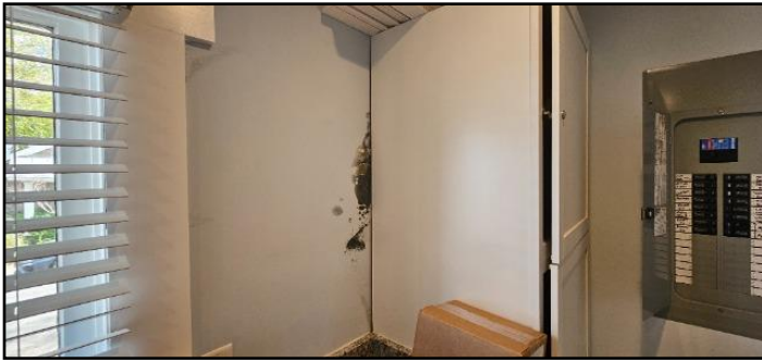
25. Visible growth on wall behind cabinet
