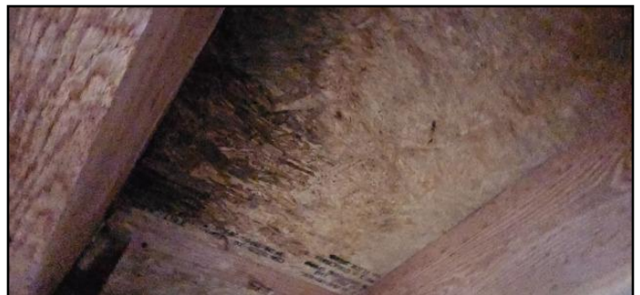
71. Wet subfloor near HVAC plenum
