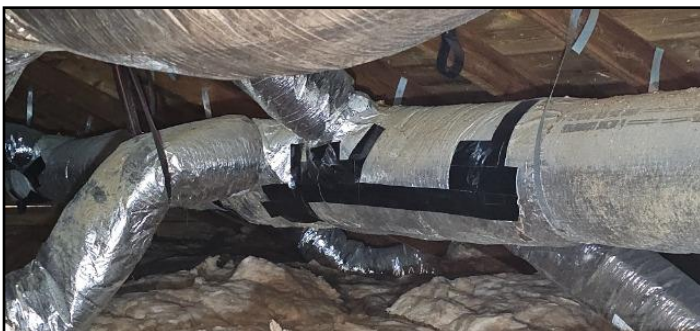
45. Ductwork repaired with improper duct tape
