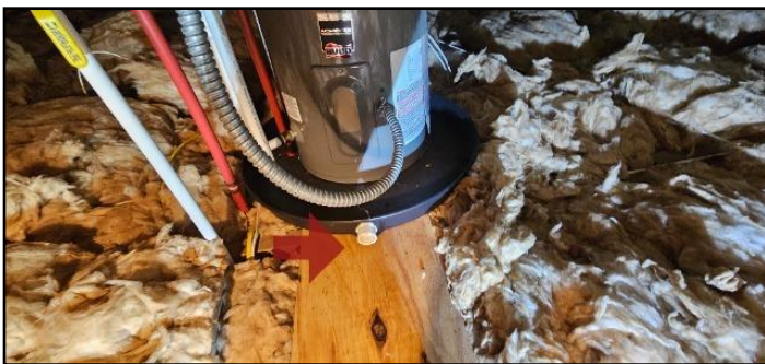
43. Drain line capped - improper
