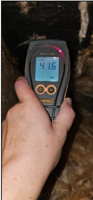
76. Wet subfloor near HVAC plenum
