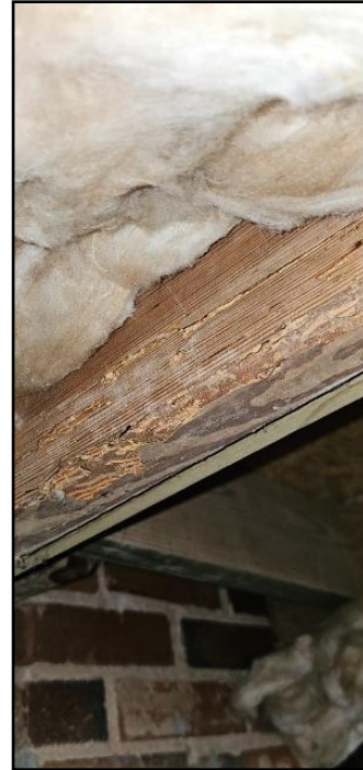
67. Visible growth on floor joists
