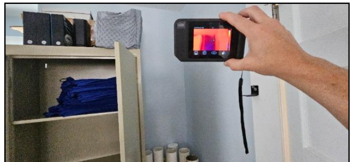
20. Moisture noted at drywall around plenum
