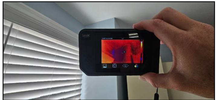
18. Moisture noted at drywall around plenum
