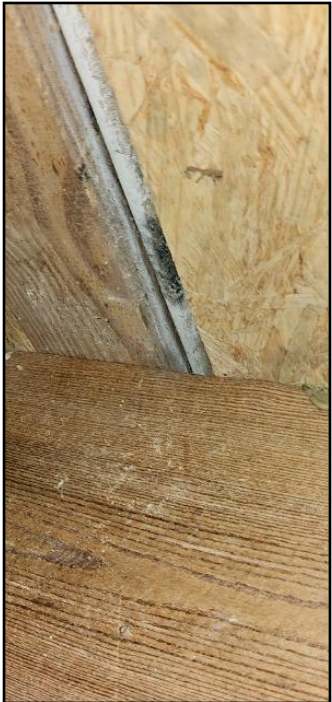
64. Microbial growth on drywall
