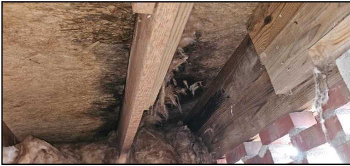
80. Water damaged subfloor
