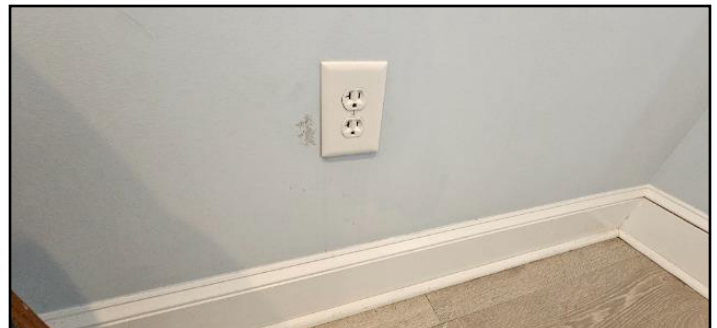
2. Visible growth at wall outlet
