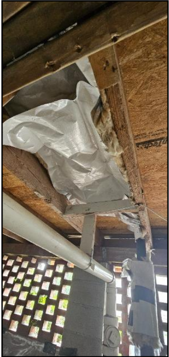
66. Plumbing access limited due to plastic
