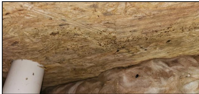
82. Visible growth on subfloor
