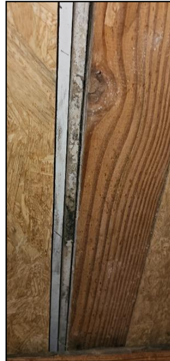
65. Microbial growth on drywall
