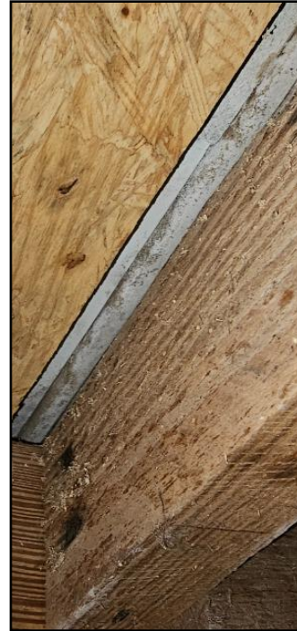
63. Microbial growth on drywall
