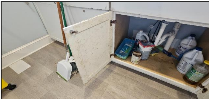
27. Visible growth on cabinets
