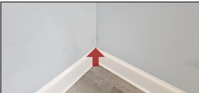
3. Visible growth at corner of wall
