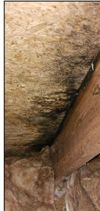
77. Wet subfloor near HVAC plenum
