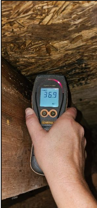
72. Wet subfloor near HVAC plenum
