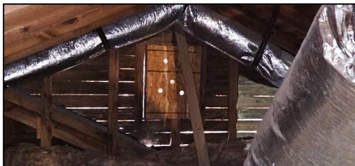
42. Gaps in siding - no wall sheathing installed
