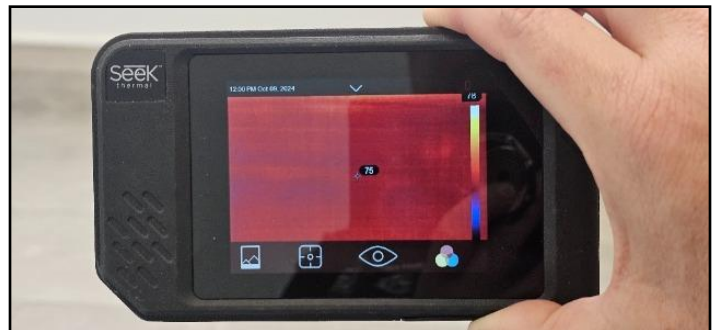
32. Moisture in wall above baseboards
