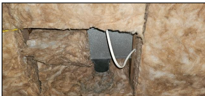
40. Exhaust fan not exhausted to exterior
