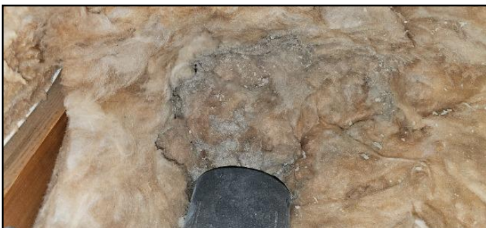
41. Discolored insulation should be removed
