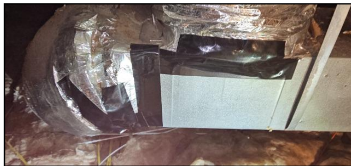
44. Ductwork repaired with improper duct tape
