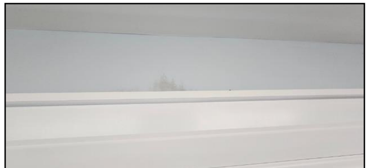
4. Visible growth or infiltration above window
