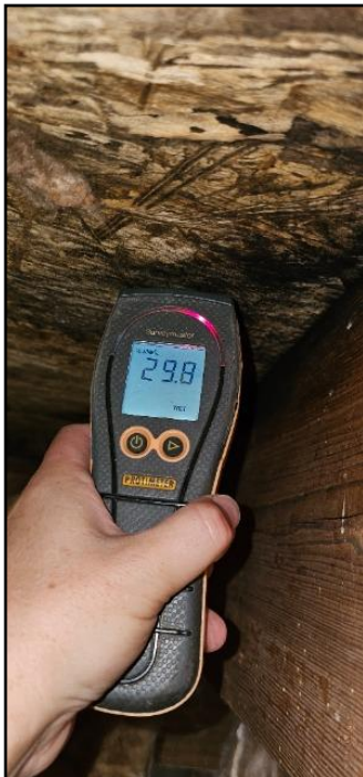
78. Wet subfloor near HVAC plenum
