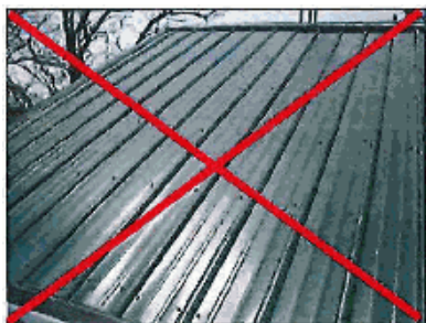
Figure 3.1.4 Inaccurate Metal Roof Example
