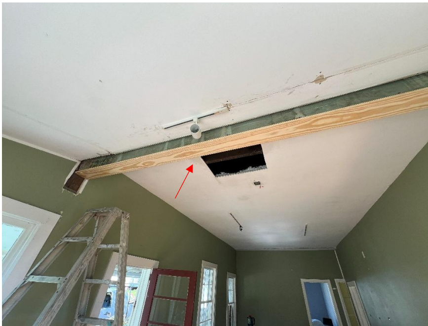
Exposed beam shows original house color
