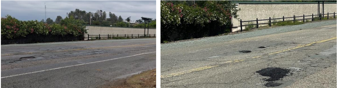
Ridge Road (Pothole first notice and fixed)
