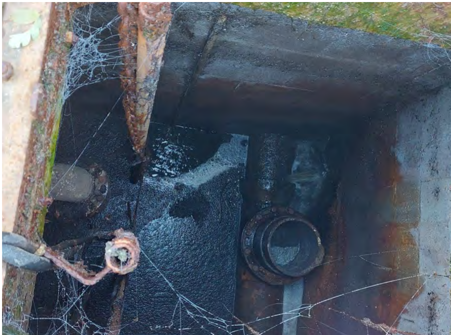
Return Valve in E-pump Vault
