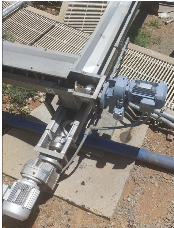
New Gear box for Headworks Auger
