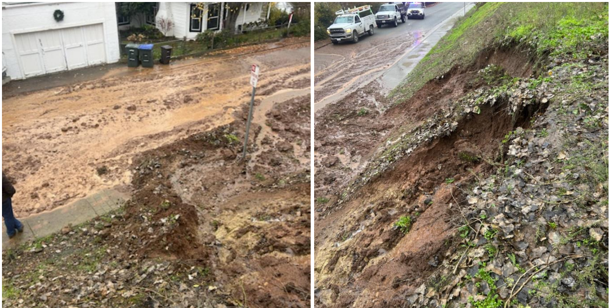
(Hillside collapse due to water leak on school property around 280 Spanish Street)
