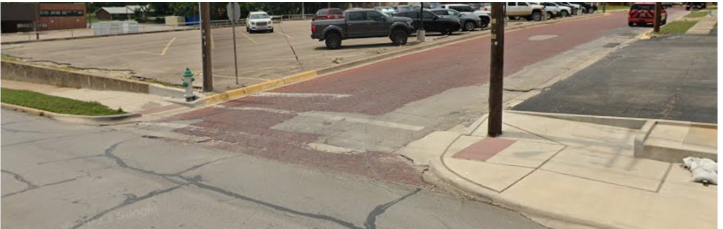
Example of sidewalk with uneven surfaces and limited ADA accessibility (corner of Washington & Barton Avenues)
