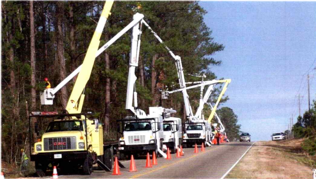
Hazard Tree Removal (Leaner)
