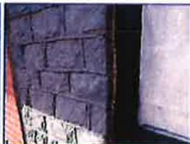
Areas of open joints around window frames
