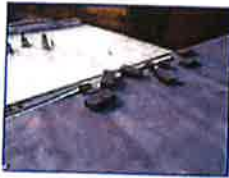
Debris on roof
