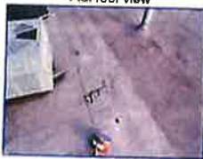
Evidence of patching on roof
