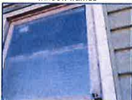
Thermal pane window fogged at right side of building
