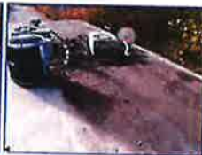
Ponding on flat roof
