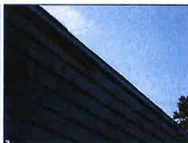
Areas of damaged/missing trim at right side of building
