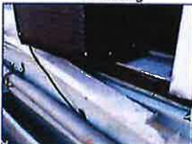
Areas of damaged window at right side of building
