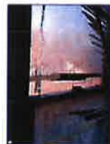
Thermal pane windows fogged at right side of building
