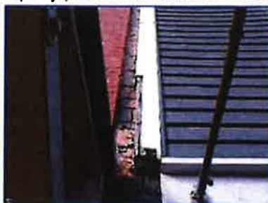
Areas of damaged/missing trim at front of building
