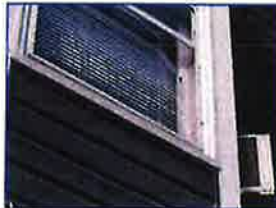
Areas of damaged window at front of building
