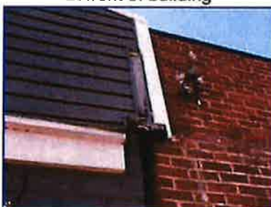
Areas of damaged trim at front of building
