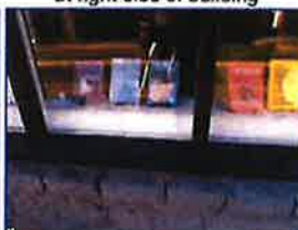
Areas of unpainted or unsealed portions of window
