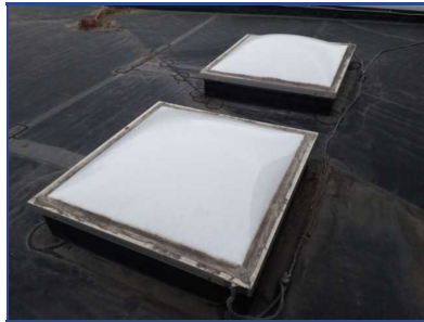
SECTION A - Def 2 - Before Photo
