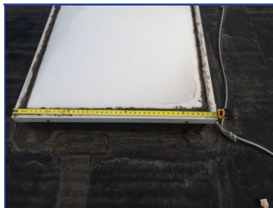
SECTION C - Def 3 - Before Photo
