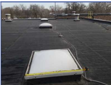
SECTION C - Def 3 - Before Photo
