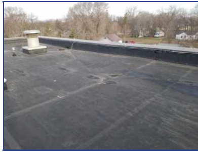
SECTION B - Def 3 - Before Photo
