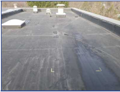
SECTION B - Def 3 - Before Photo
