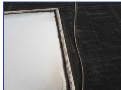
SECTION C - Def 3 - Before Photo
