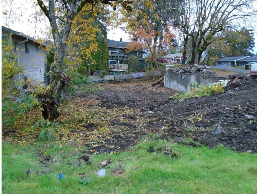
Left: November 2024 of the subject property a seen from Wyeth Street following demolition of the building. Note the foundation wall and grade difference.
