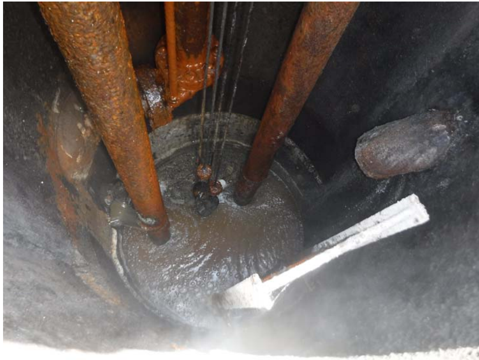
Figure 2. Kanaka Pump Station Wetwell. LDB Beverage sample location will be from a container suspended below the influent sewer shown on right.
