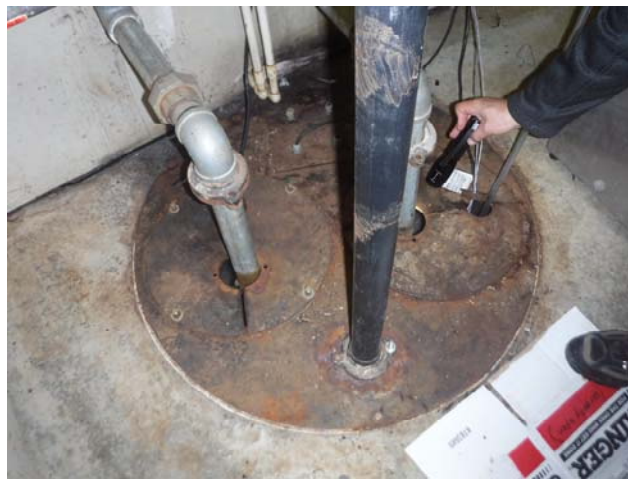
Figure 1. Sampling location for the Waterfront Building. Sump is located below the metal cover. Metal pipes shown are sump pump discharge lines, and plastic pipe is an influent drain line.
