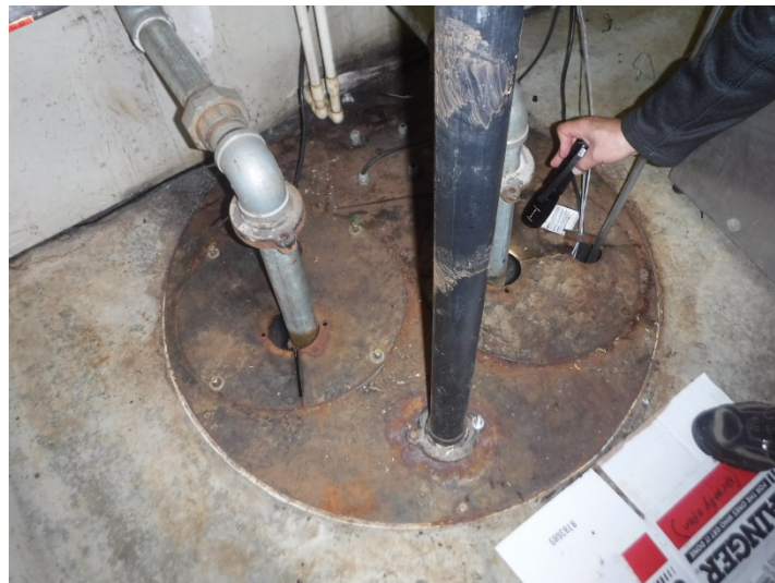
Figure 1. Sampling location for the Waterfront Building. Sump is located below the metal cover. Metal pipes shown are sump pump discharge lines, and plastic pipe is an influent drain line.
