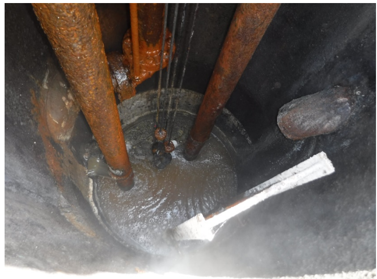
Figure 2. Kanaka Pump Station Wetwell. LDB Beverage sample location will be from a container suspended below the influent sewer shown on right.
