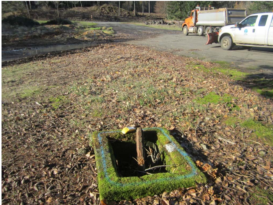
Photograph 2: Water valve feature in central portion of Property. Photograph taken facing west.
