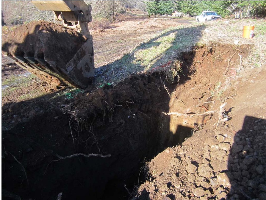
Photograph 5: Excavation of TP6 within the footprint of the southern former wigwam burner. The shelf feature in the photograph is a concrete slab encountered during advancement of the test pit. Photograph taken facing northwest.
