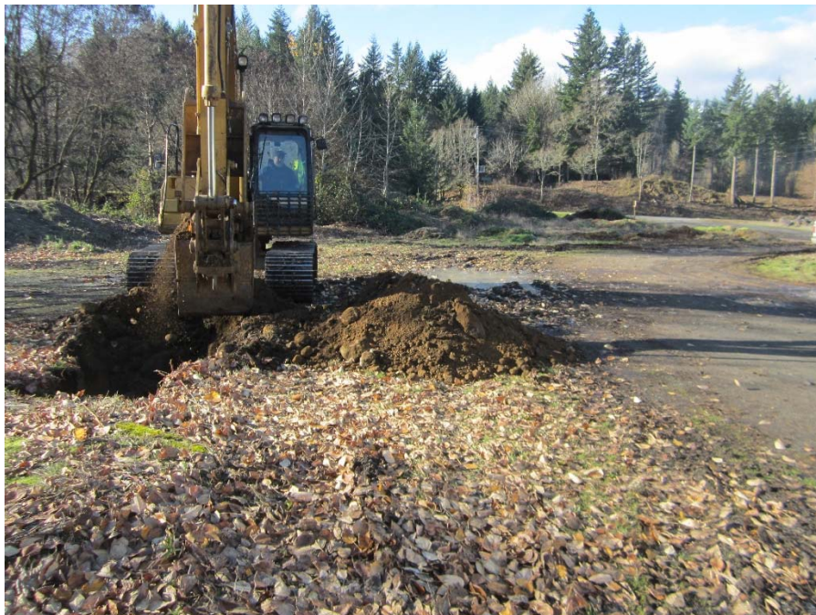
Photograph 6: Excavation TP8 adjacent to the northeast corner of the small structure foundation. Photograph taken facing west.
