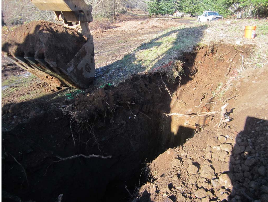
Photograph 5: Excavation of TP6 within the footprint of the southern former wigwam burner. The shelf feature in the photograph is a concrete slab encountered during advancement of the test pit. Photograph taken facing northwest.
