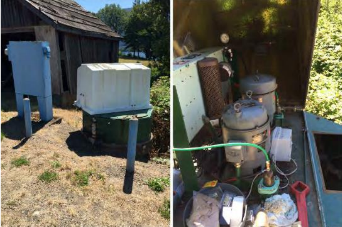
Figure 2-2 Cascade Pump Station Photos
