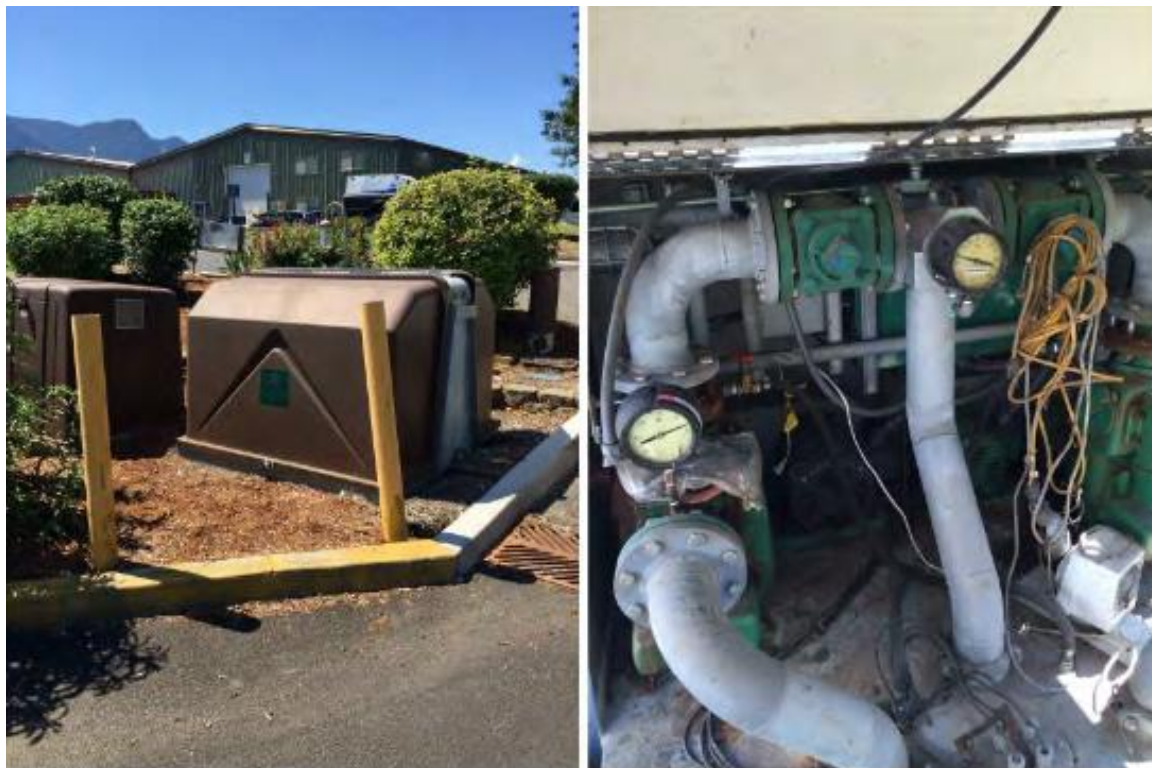
Figure 2-3 Kanaka Creek Pump Station Photos
