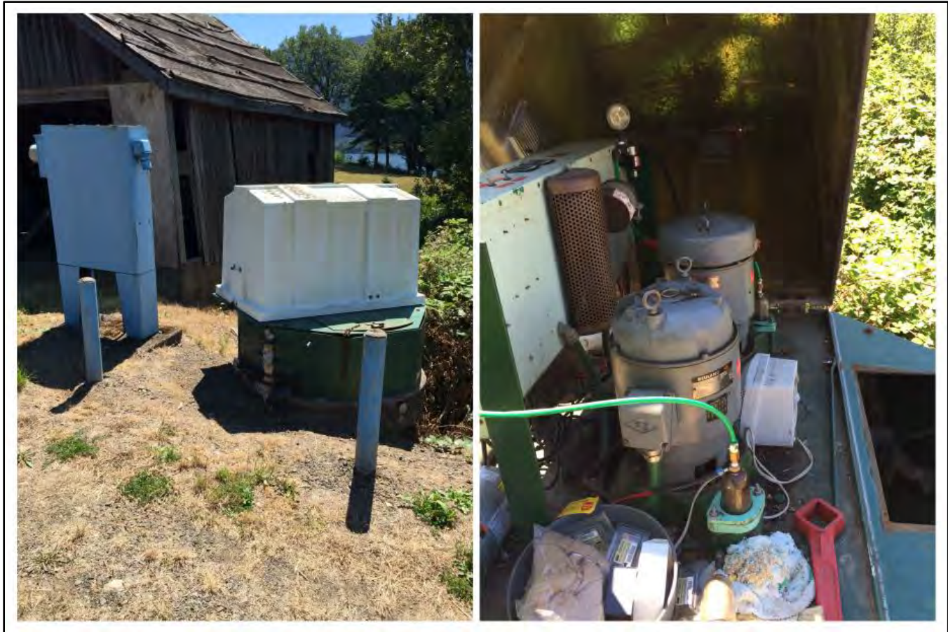
Figure 3-7. Cascade Pump Station Photos
