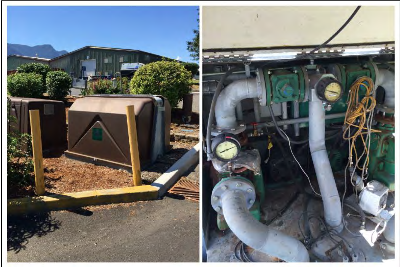
Figure 3-6. Kanaka Pump Station Photos
