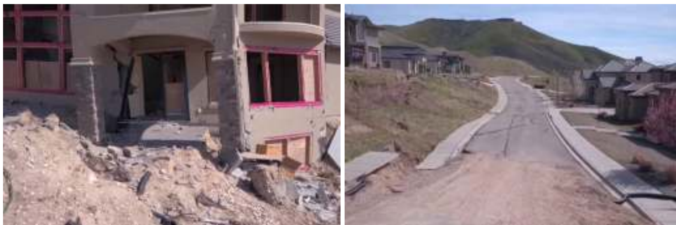
Figure 16-2. Residential and Infrastructure Damage, Alto Via Court
