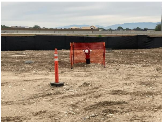
FIGURE 8-6B-3(a) HYDRANT FENCING
