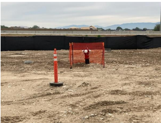
FIGURE 8-6B-3(a) HYDRANT FENCING
