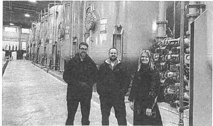
Jim Westerman and Jason Egerstrom from the city of Woodbury with Alycia Overbo of MDH in front of the GAC filters.
