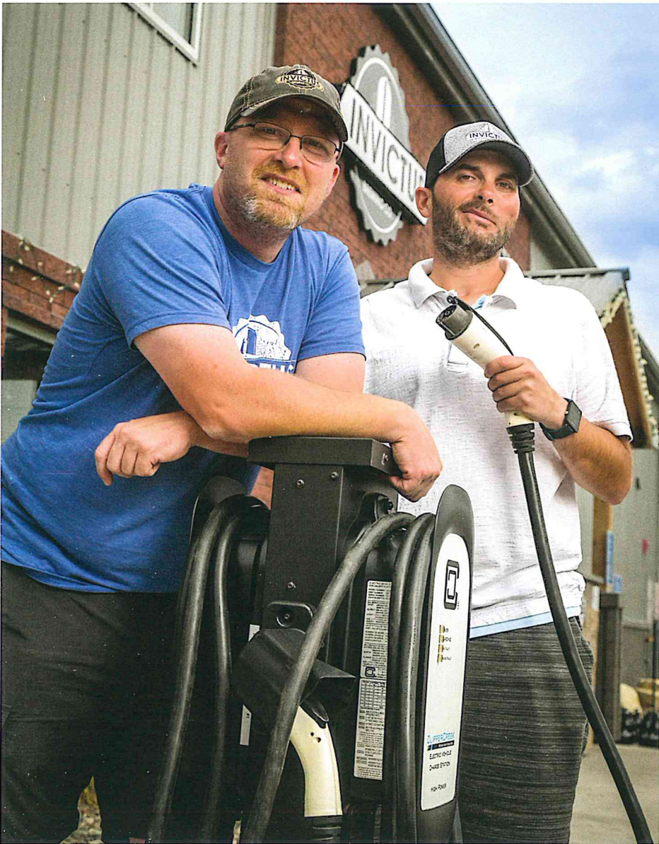
Six electric vehicle chargers are installed by the front doors. And, while Previn Solberg and Sam Villella admit they will not be making any money on the chargers, they feel good about giving that energy back to the community.
