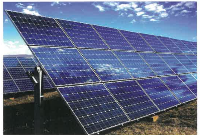
Xcel Energy's Sherco Project is planned to be completed in 2025. Xcel Energy file photo.
