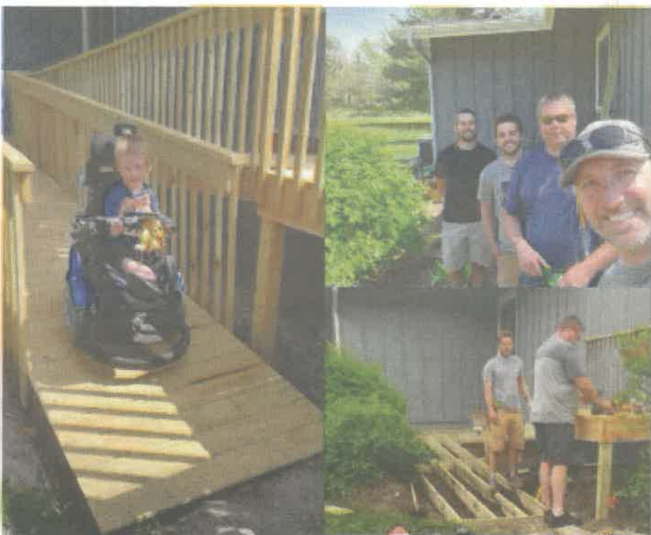
Vujovich designed and remodeled a deck to give a family's son the flexibility to exit the home through the front door or the back door
