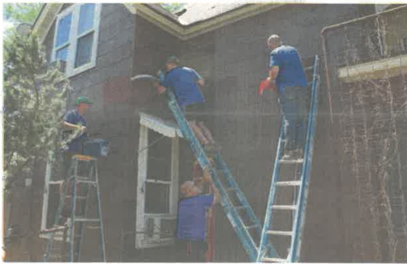
Creative Homes employees painted, landscaped, cleaned the yard, and assisted with exterior home repairs.
