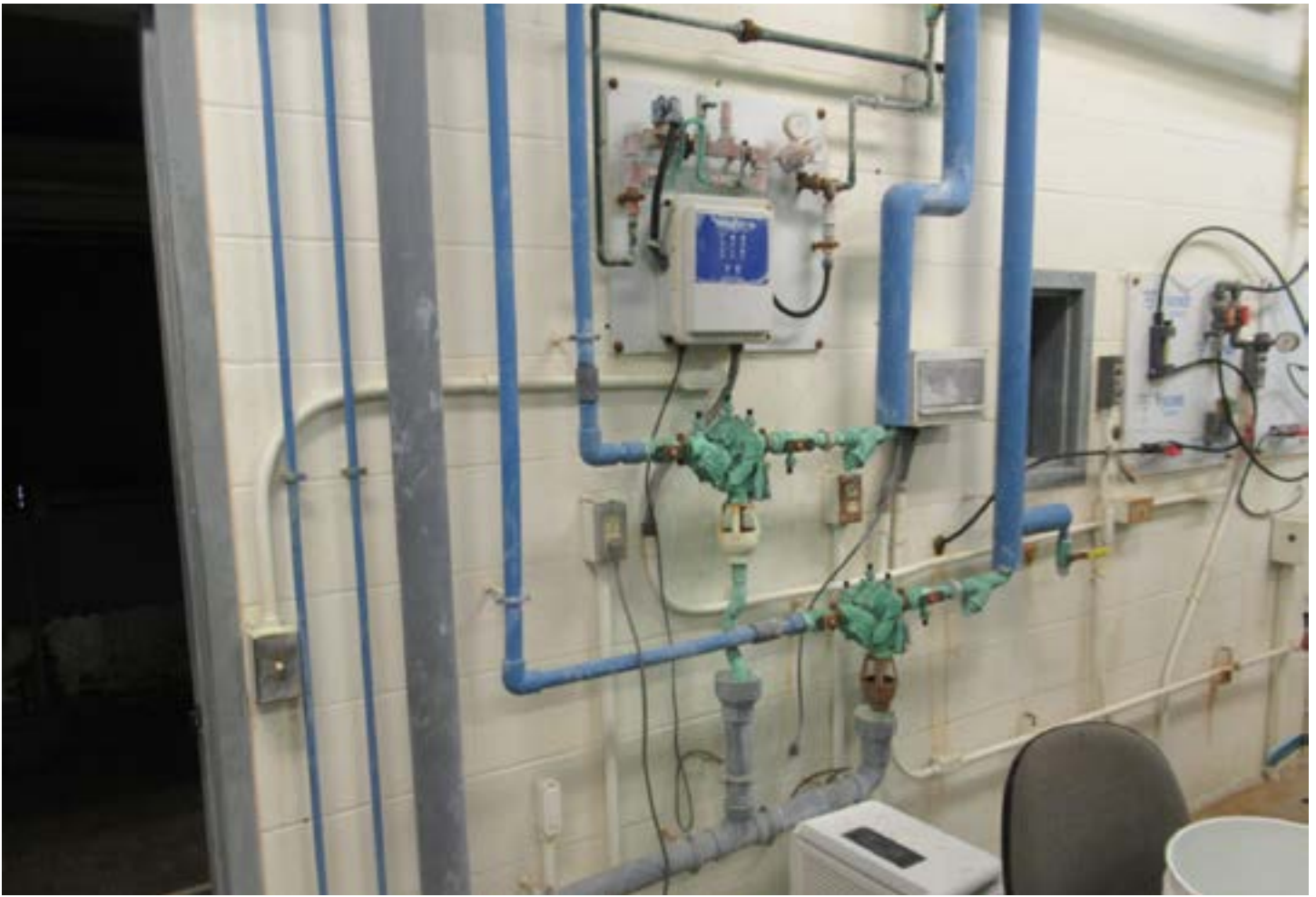
The chlorine leak caused damage to the backflow preventers that serve the water supply to the chlorine feed systems.
