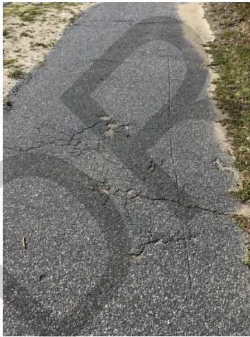
Figure A - Transverse Cracking
