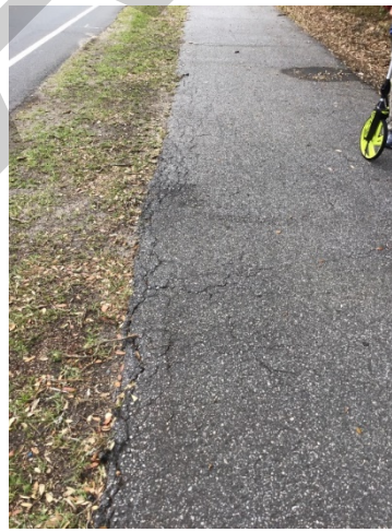
Figure B – Edge Cracking
