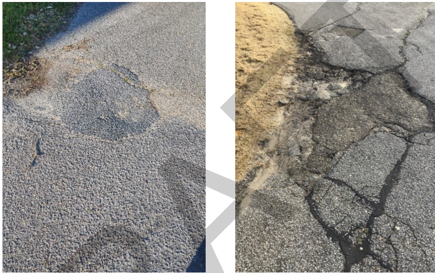
Figures 7 & 8: Patching that is failing (patches sinking and cracking)
