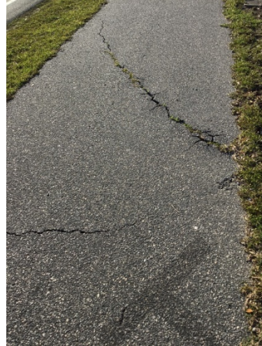
Figure D – More cracking due to roots
