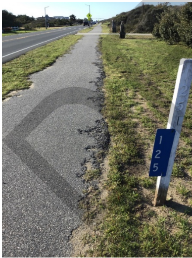
Figure E – Raveling of asphalt edges
