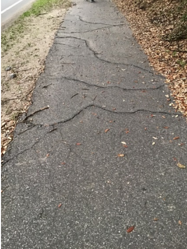
Figure C – Root intrusion cracks
