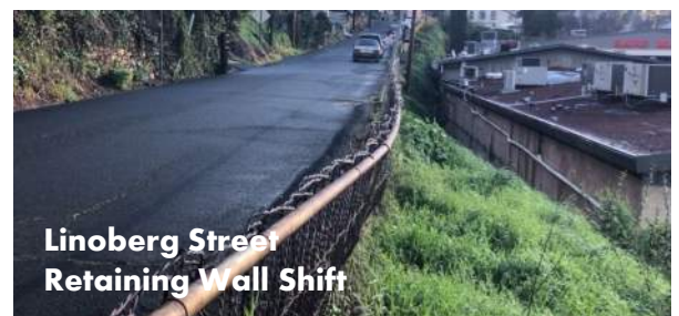
Linoberg Street Retaining Wall Erosion
