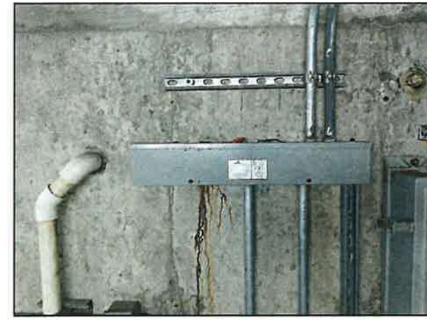
EXISTING FLOOD SWITCH JUNCTION BOX
