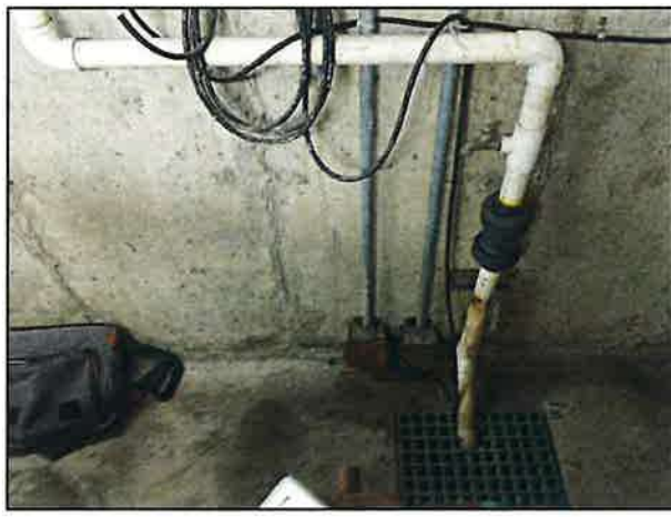
EXISTING FLOOD SWITCHES AND SUMP.
