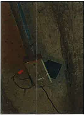
EXISTING PRESSURE TRANSMITTER JUNCTION BOX
