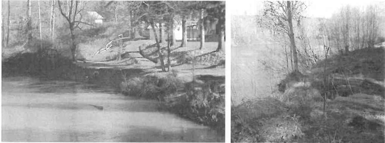
Figure 3: 2007 Photos of Bank Erosion near Sewer Pipe upstream of Meadowbrook Bridge at Walnut Street
