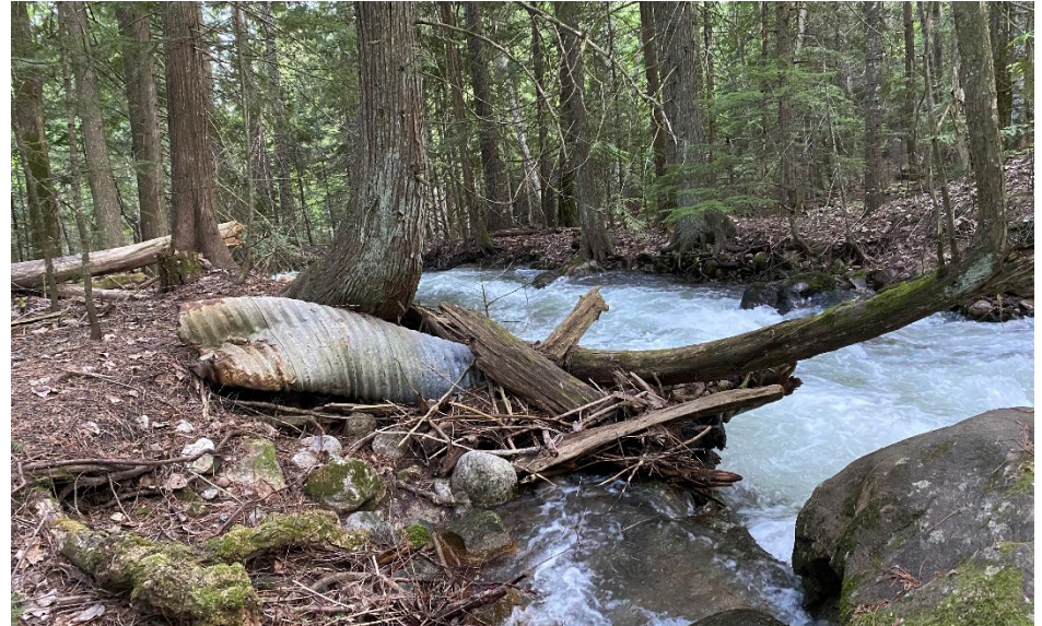
Damaged culvert located on lower portion of Little Sand Creek shows need for protection and remediation along creek to protect water quality.
