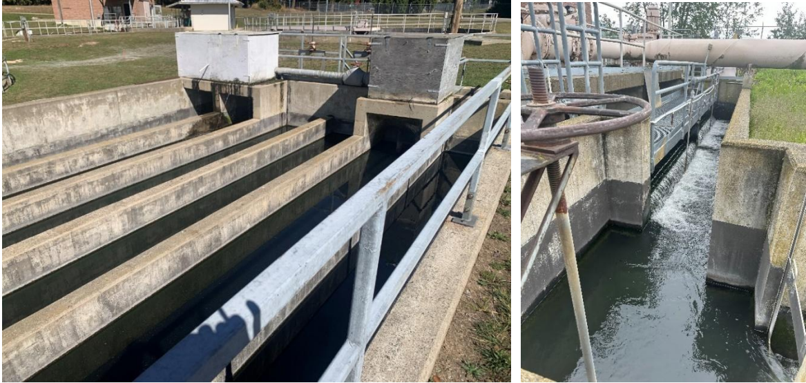
FIGURE 2-13: CHLORINE CONTACT BASIN AND EFFLUENT CHANNEL
