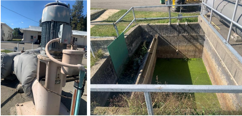
FIGURE 2-6: OVERFLOW PUMP AND DETENTION TANK
