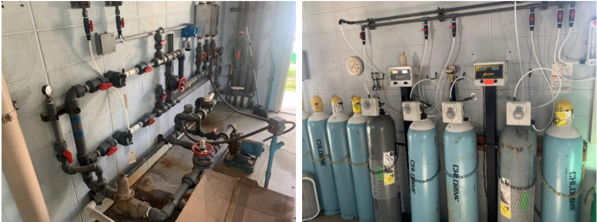
FIGURE 2-14: CHLORINE FEED SYSTEM AND STORAGE
