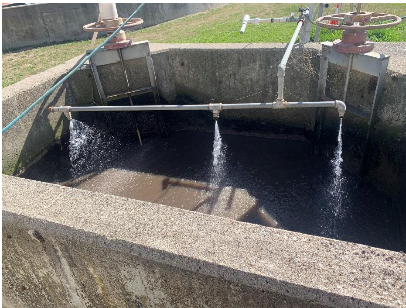
FIGURE 2-11: CLARIFIER SPLITTER BOX
