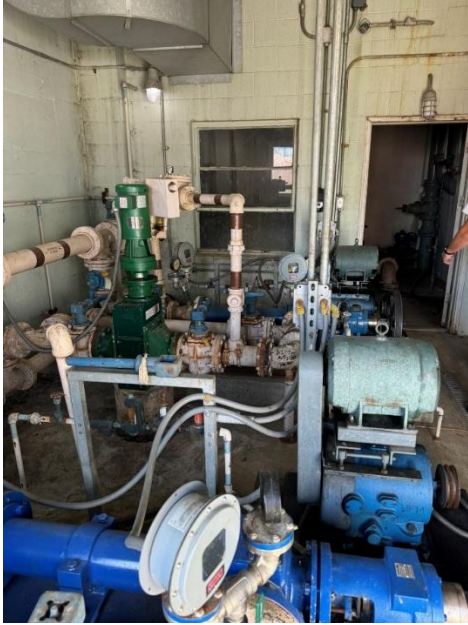
FIGURE 2-18: DIGESTED SLUDGE TRANSFER PUMPS
