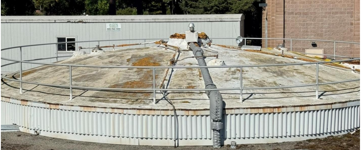
FIGURE 2-19: ANAEROBIC DIGESTER EXTERIOR
