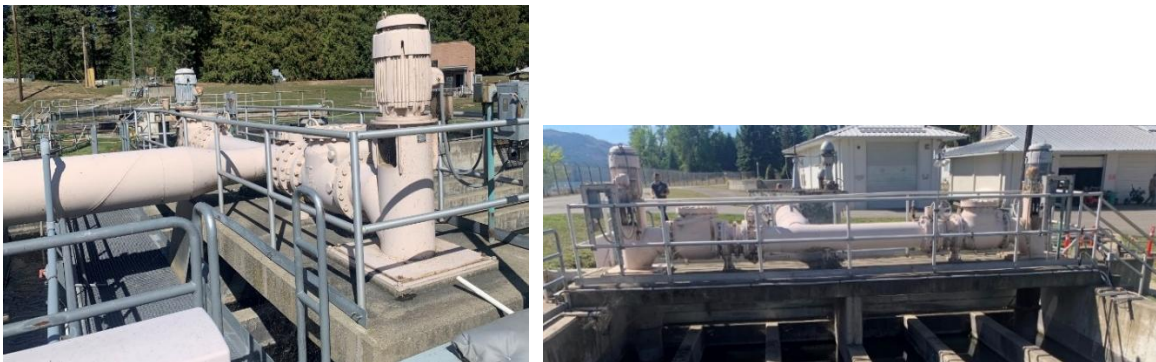
FIGURE 2-15: FLOOD STAGE PUMPS
