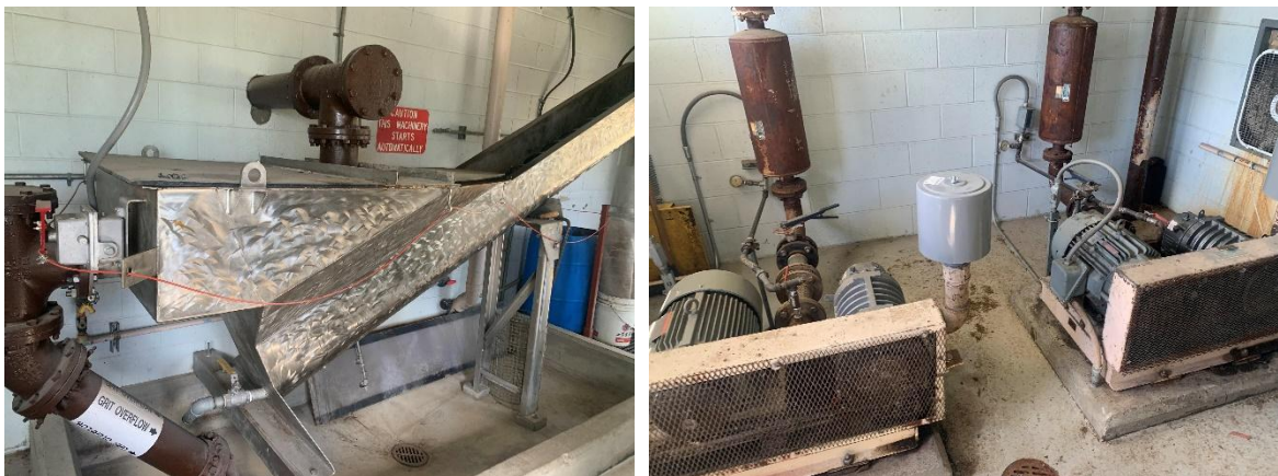
FIGURE 2-2: GRIT CLASSIFIER AND BLOWERS
