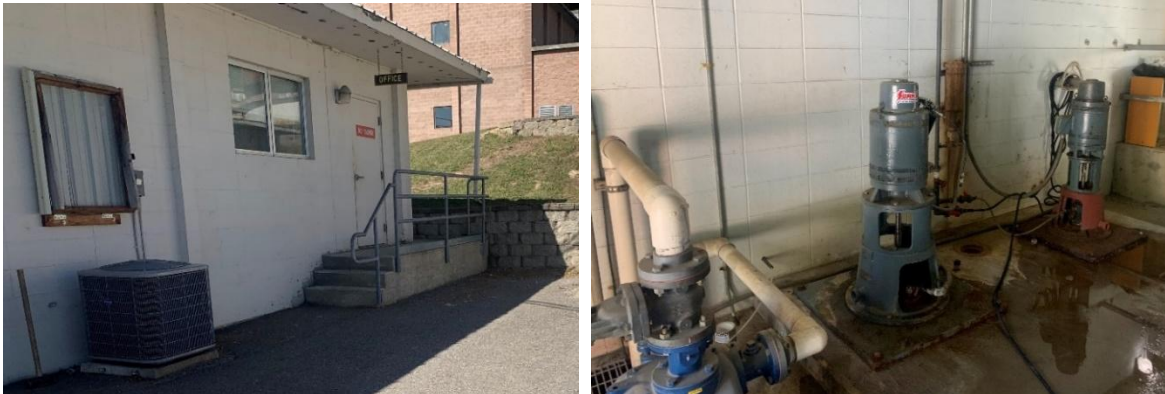
FIGURE 2-7: SECONDARY CONTROL BUILDING AND INTERMEDIATE PUMPS
