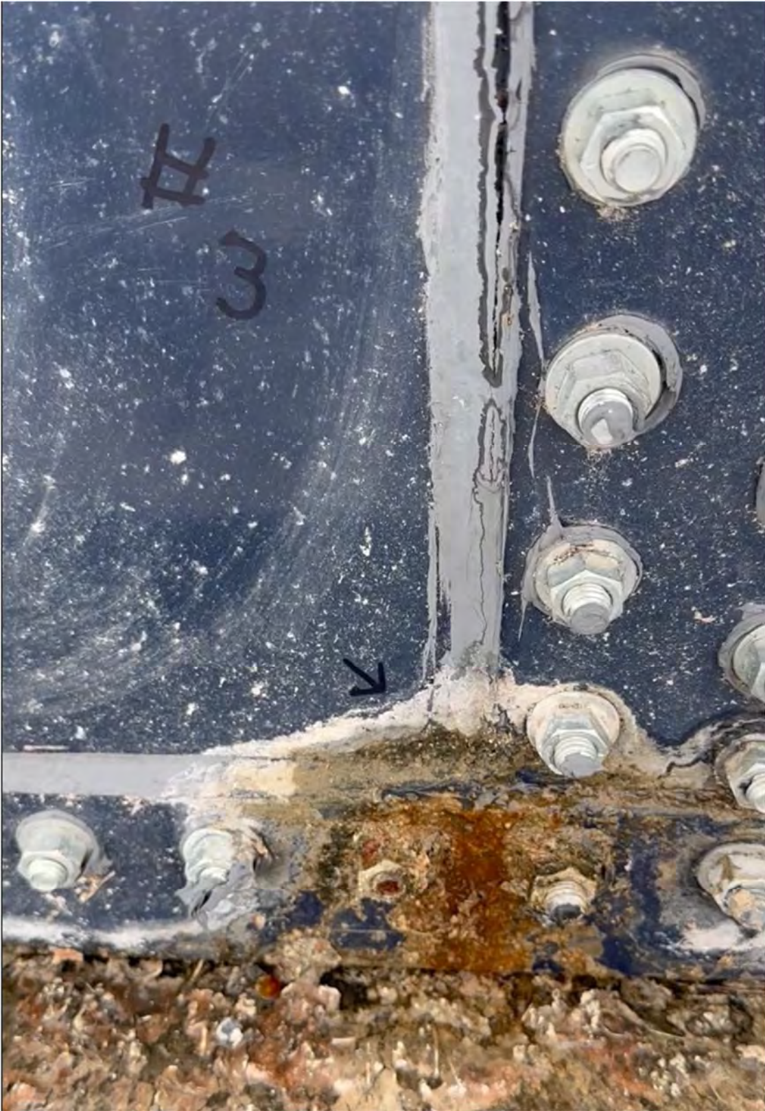
FIGURE 3 - LEAK 3, LOCATION OF PREVIOUS AND EXISTING LEAK
