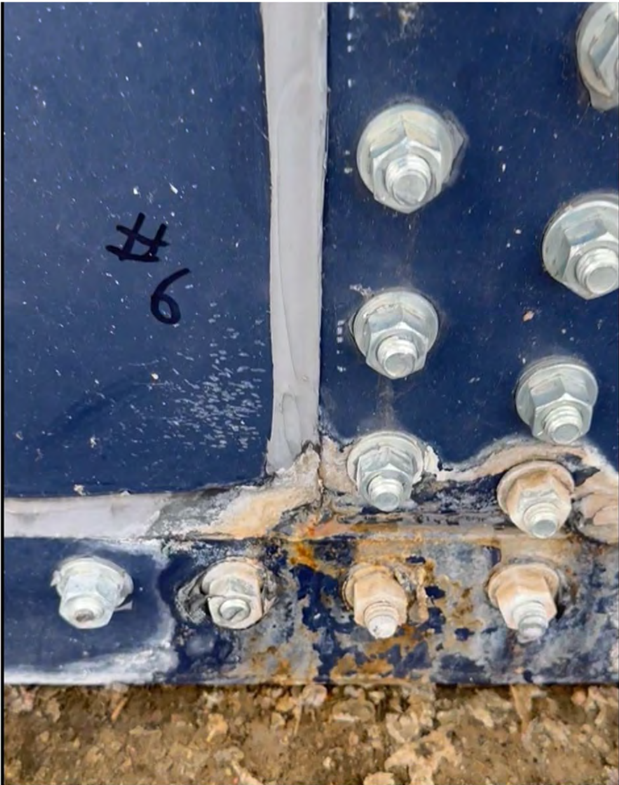
FIGURE 6 - LEAK 6, FLOWING LEAK
