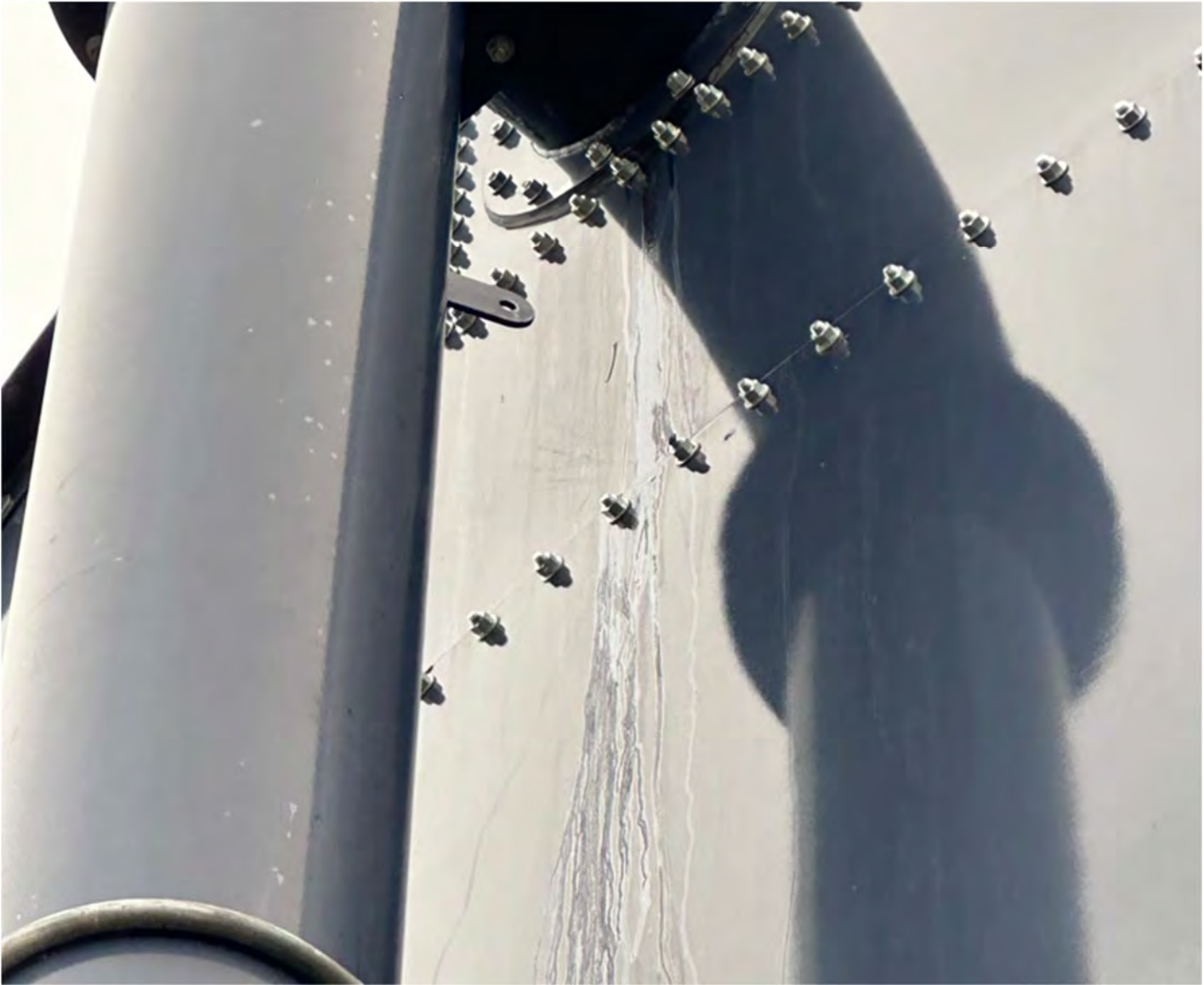
FIGURE 12 - LEAK 12, OVERFLOW PIPE
