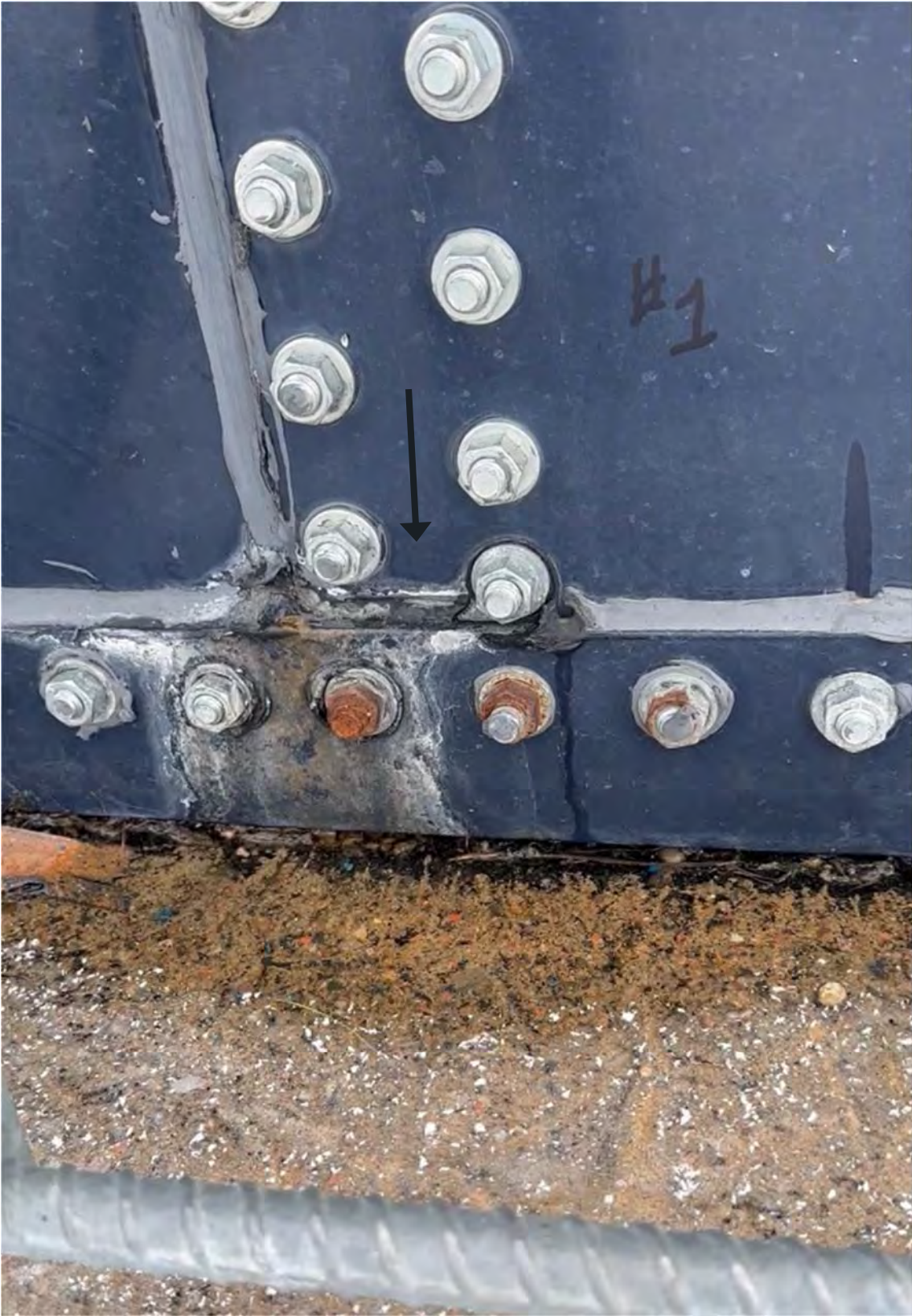
FIGURE 1 - LEAK 1, LOCATION OF PREVIOUS AND EXISTING LEAK
