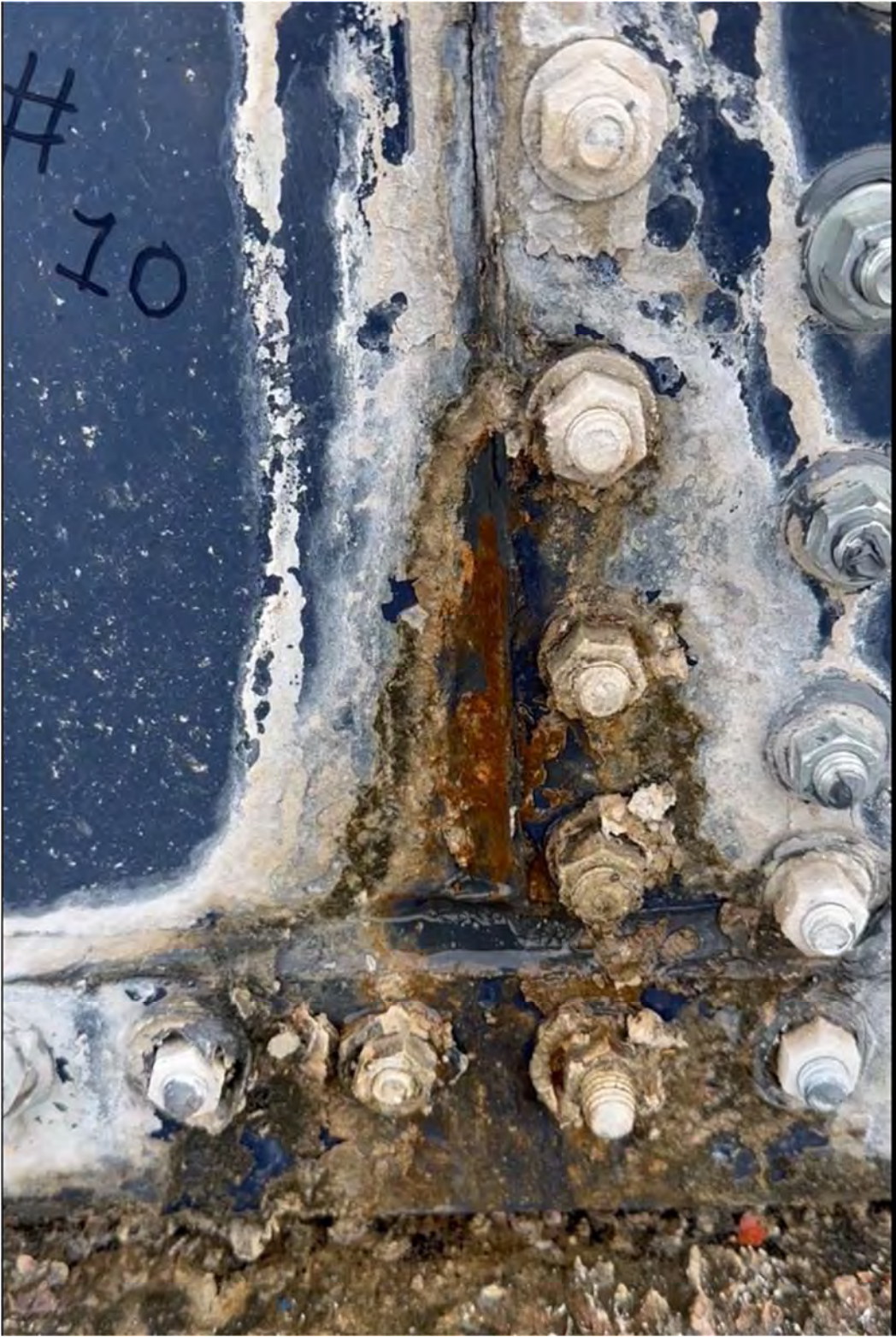
FIGURE 10 - LEAK 10, PREVIOUS AND EXISTING LEAK
