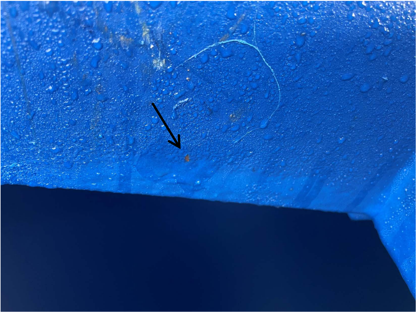
FIGURE 16 - INTERIOR BLEMISH, RUST ON TOP HATCH CURB
