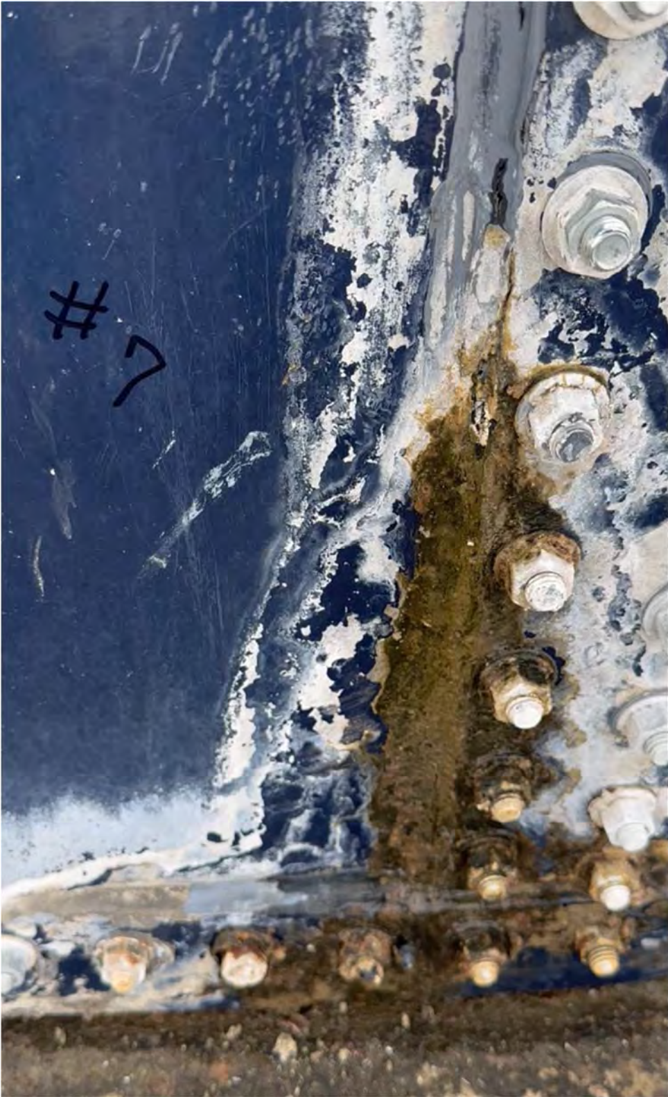
FIGURE 7 - LEAK 7, LEAK AT SEAM
