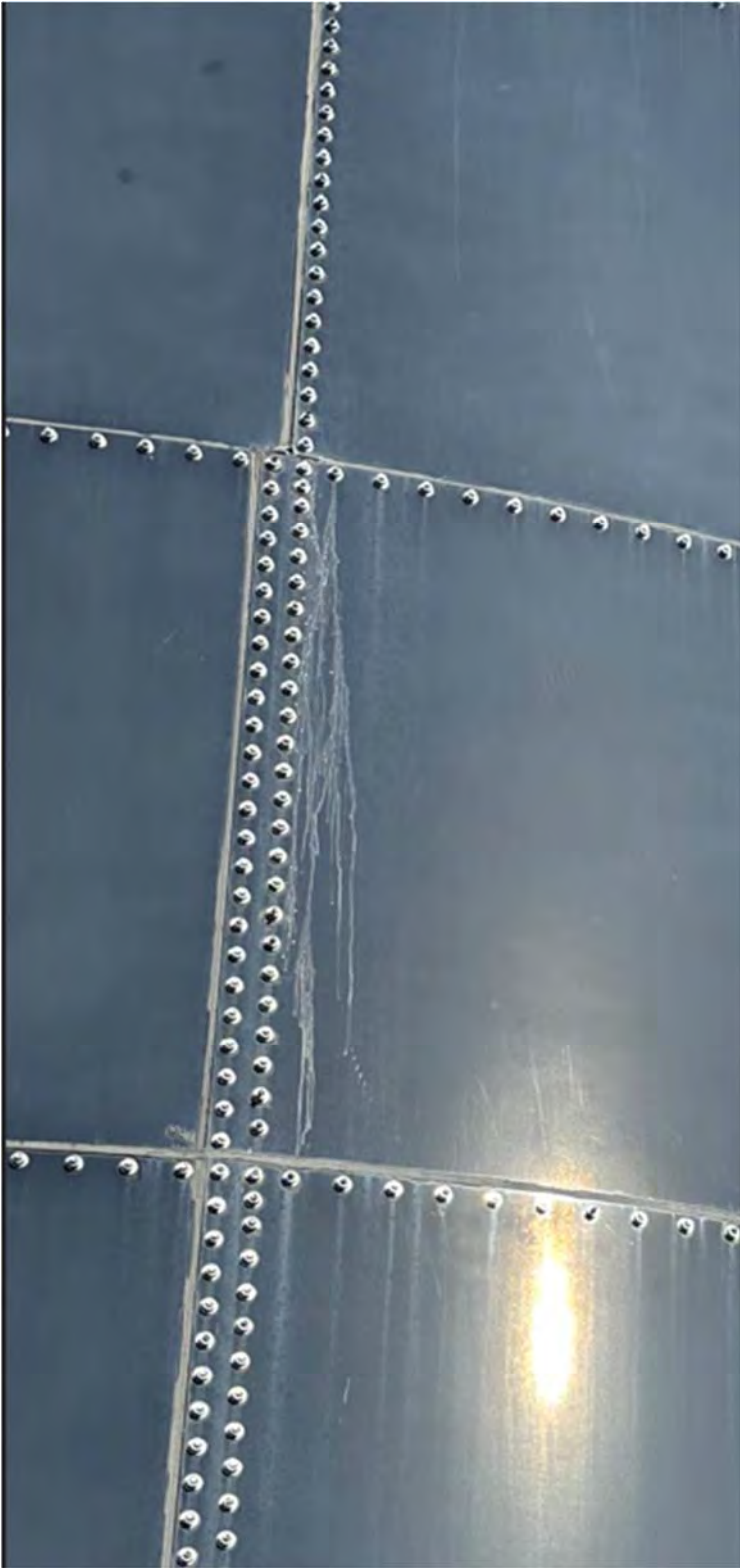
FIGURE 13 - LEAK 13, FROM BOLT HOLES
