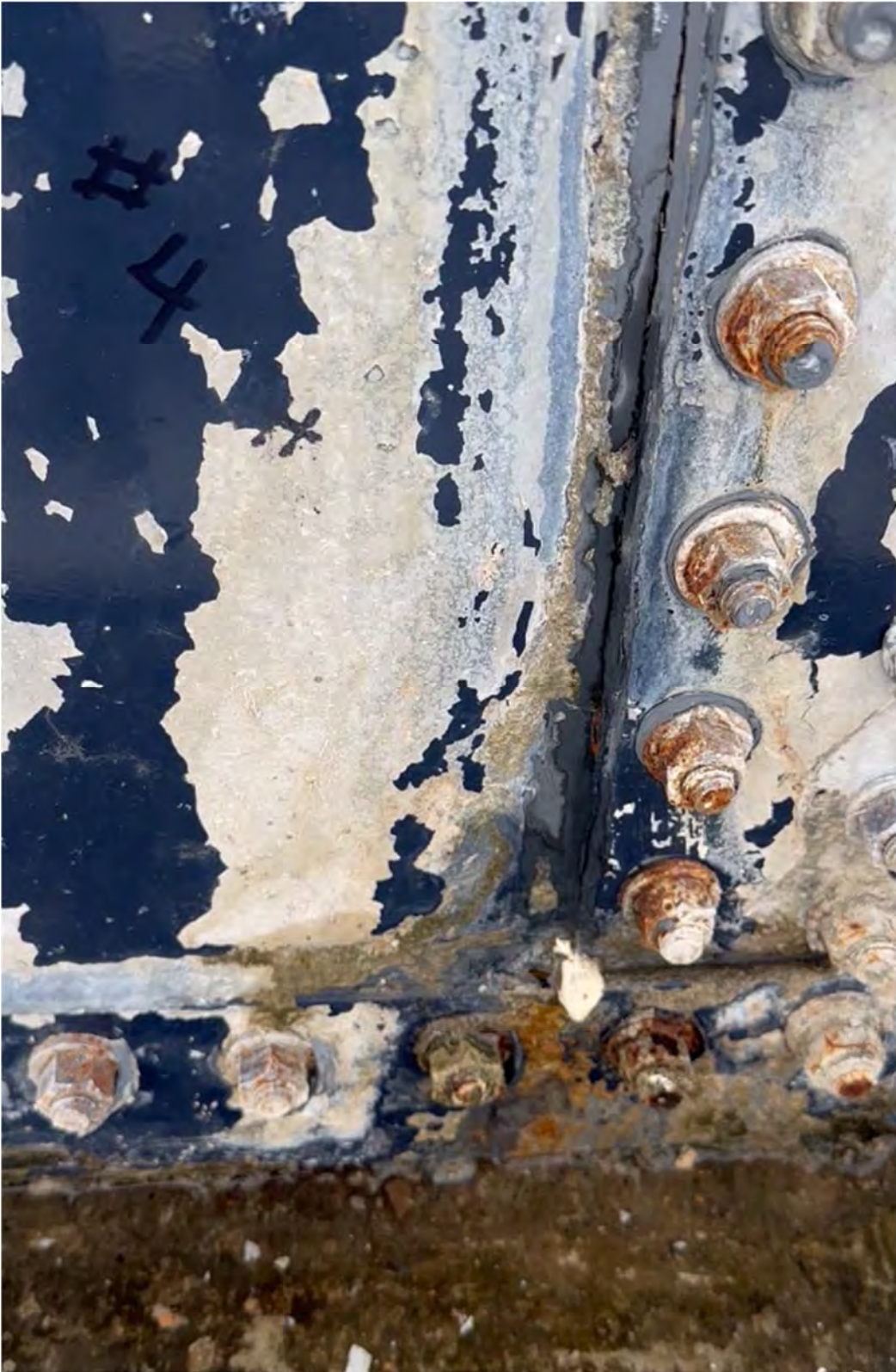
FIGURE 4 - LEAK 4, LOCATION OF PREVIOUS AND EXISTING LEAK
