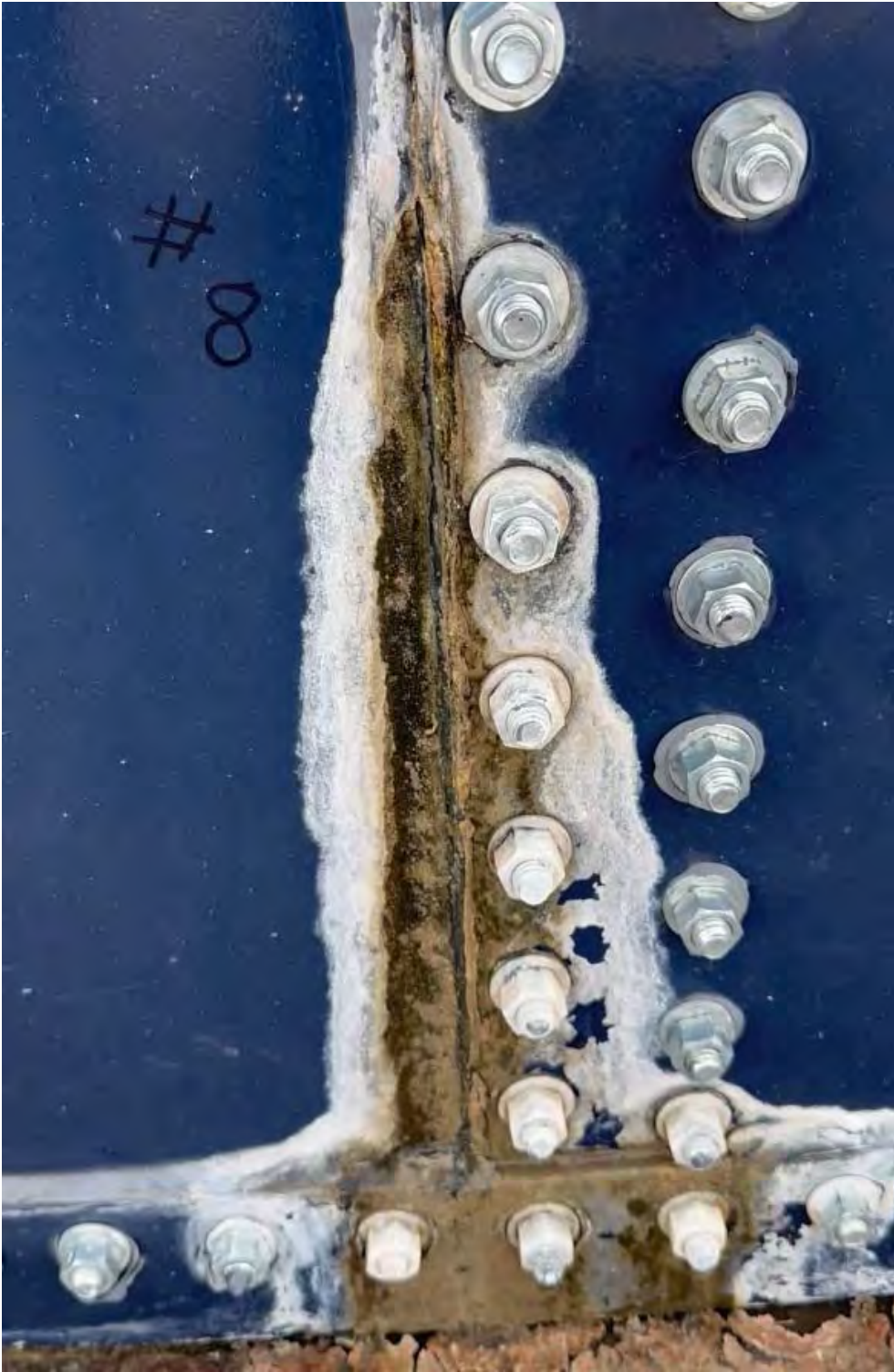
FIGURE 8 - LEAK 8, PREVIOUS AND EXISTING LEAK
