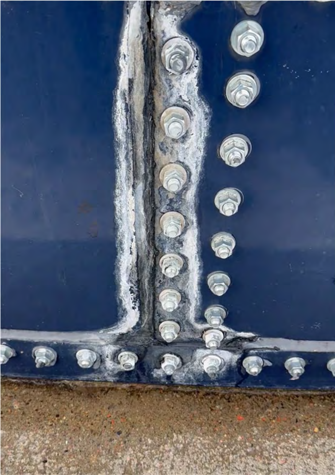
FIGURE 5 - LEAK 5, LOCATION OF PREVIOUS AND EXISTING LEAK
