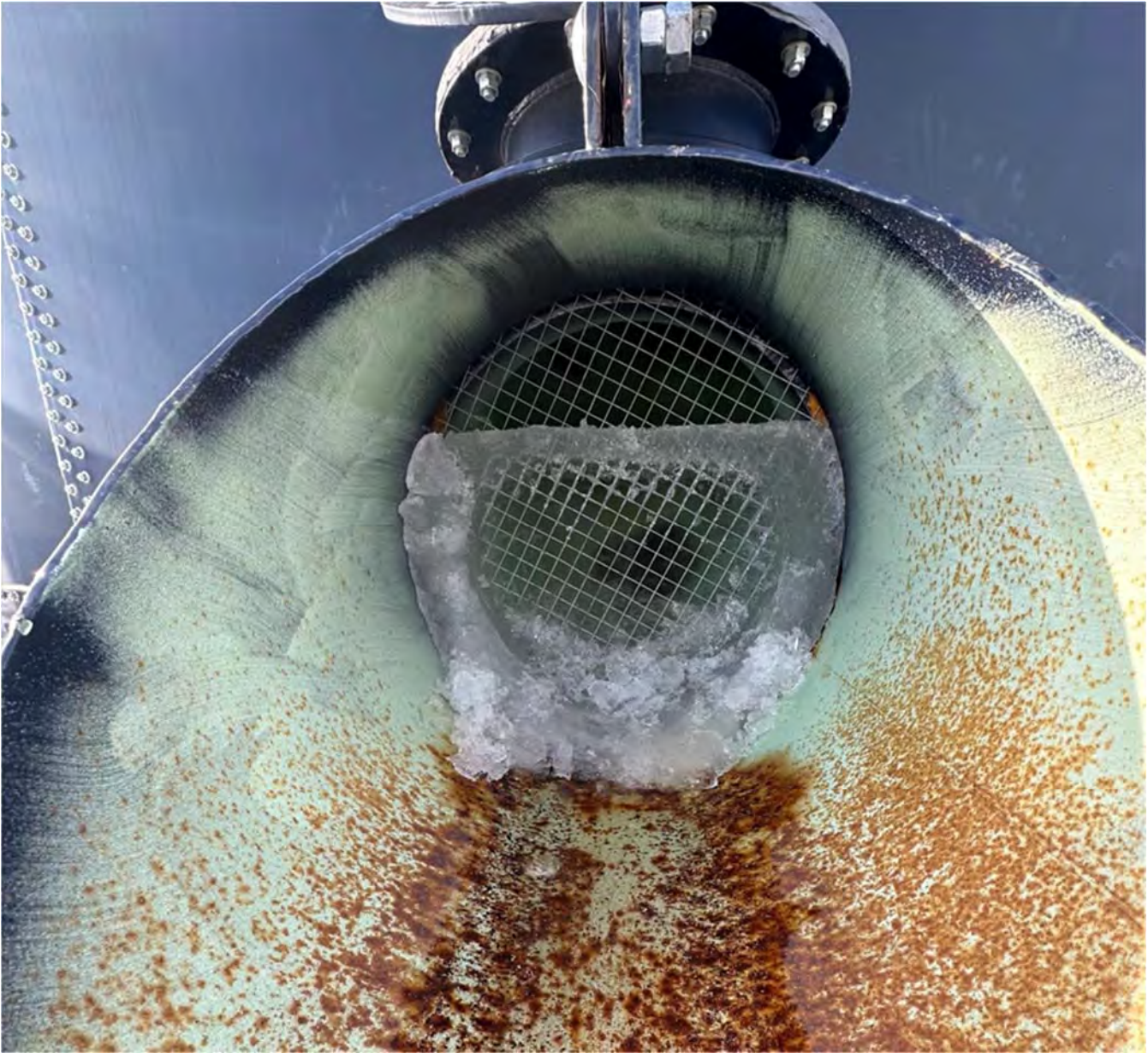
FIGURE 14 - OVERFLOW PIPE OUTLET ICE BUILDUP
