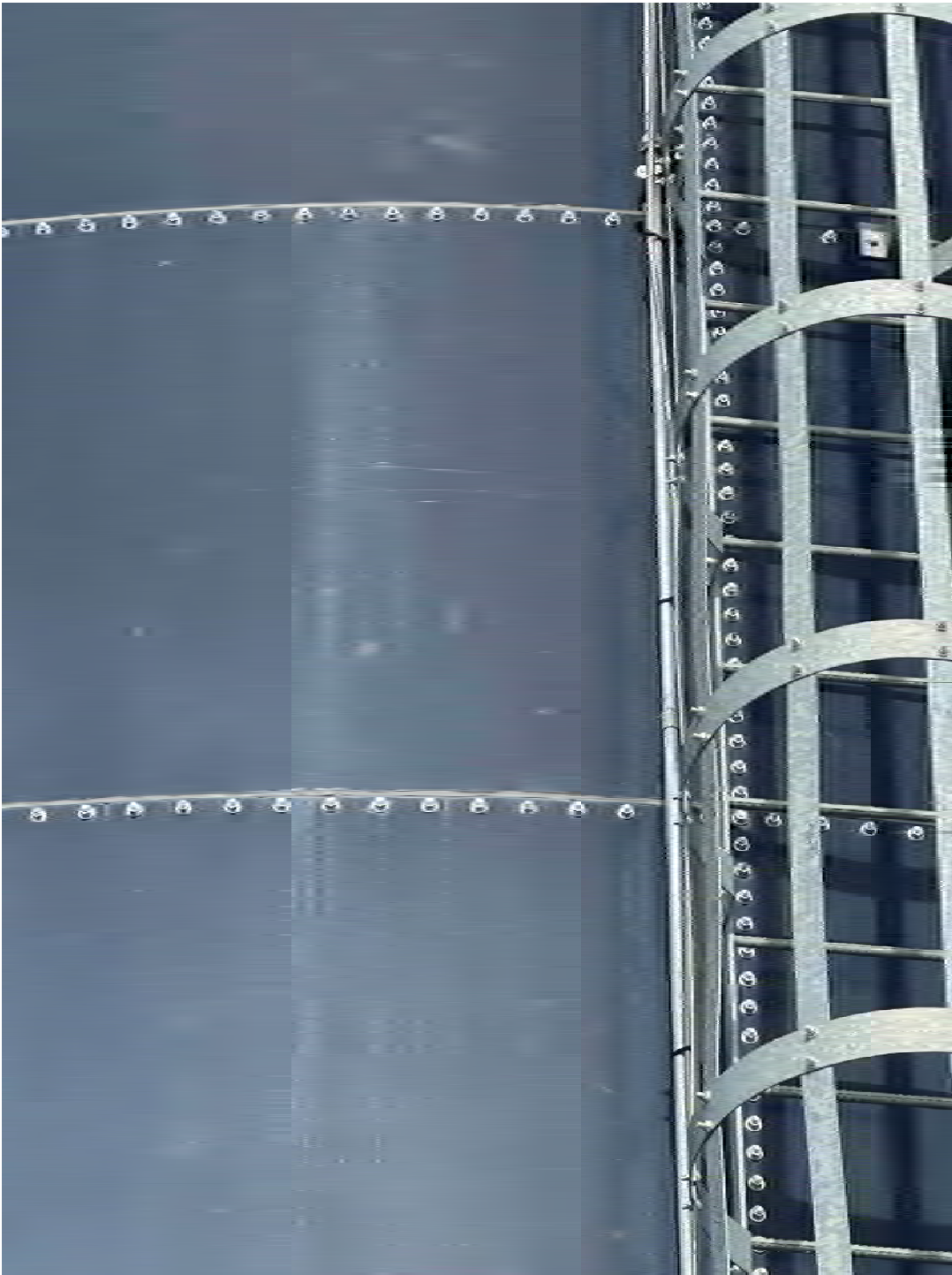
FIGURE 11 - LEAK 11, NEW LEAK FROM BOLTS
