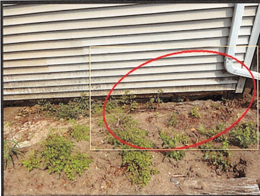
Jamie McDonald 1:13 PM Yesterday Mud sill rot from exterior
