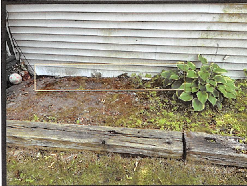
Jamie McDonald 1:12 PM Yesterday Exterior flowers beds compromising wood structure and allowing water to flow inside basement
