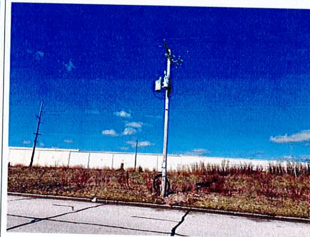
EXISTING POWER POLE / TRANSFORMER
