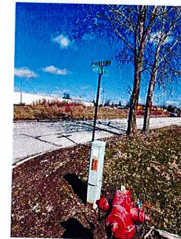
EXISTING FIBER PEDESTAL
