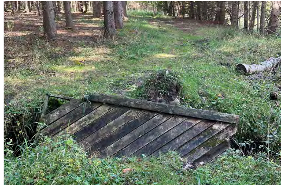
Damaged and downed bridges were documented as part of the assessment process.
