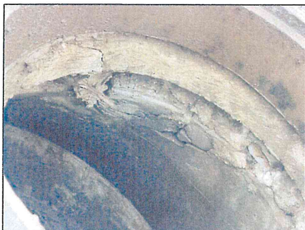
Image 5 – Connection Chimney and cone
