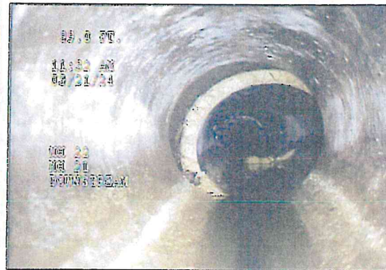
MH 22 to MH 21, offset at joint
