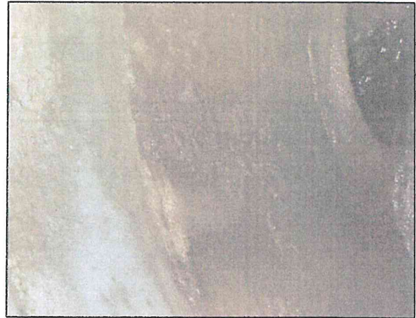
Image 4 – Connection 2, joint infiltration
