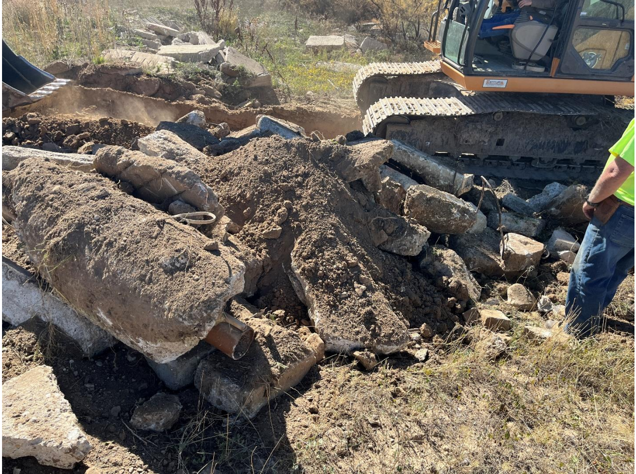
Looking south at trench between Hole 3 and Hole 4. Surface concrete and rebar pile scraped to side to dig down 10 feet and verify that there is not something buried below the surface piles.
