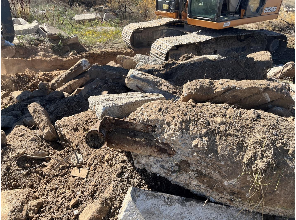
Looking south at trench between Hole 3 and 4. Note some rebar and metal gate post embedded. All material scraped at surface.
