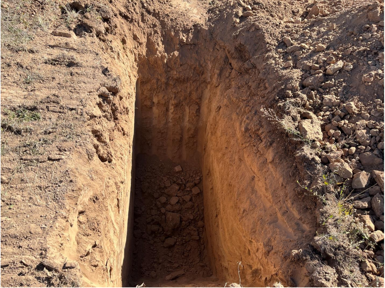
Hole 1 on Pipeline Centerline. Uniform sandy silt to 10 feet deep (pipeline invert)
