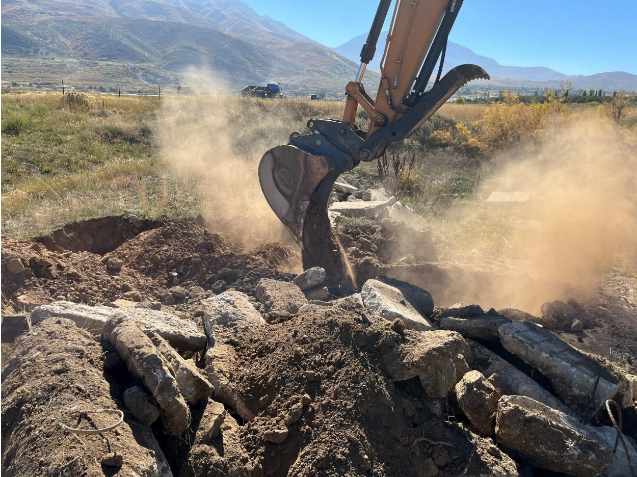
Filling trench between Holes 3 and 4. All surface debris left on surface for construction contractor to remove.
