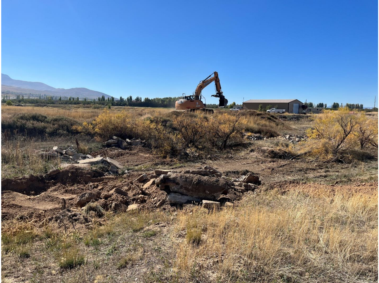
Looking west-southwest at Hole 7 location on higher filled ground south of federal easement determined to be imported topsoil. Holes 3, 4 and 5 in mid area of photo with surface debris in temporary easement scraped in piles.
