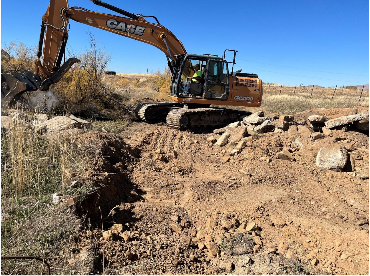
Looking west-northwest at the start of Hole 5. Trench between Holes 2 and 3 that are backfilled is shown.
