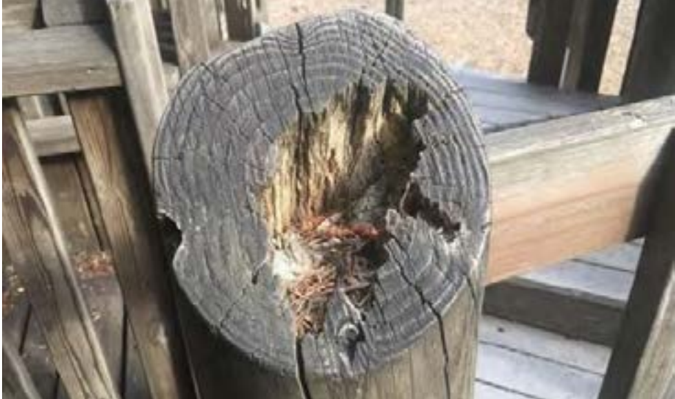
1. Splintering and declining wood frame
