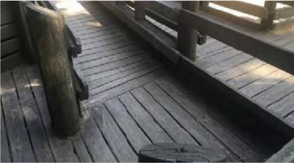
6. The current ADA accessible path is deteriorating, with visible signs of splitting and rot
