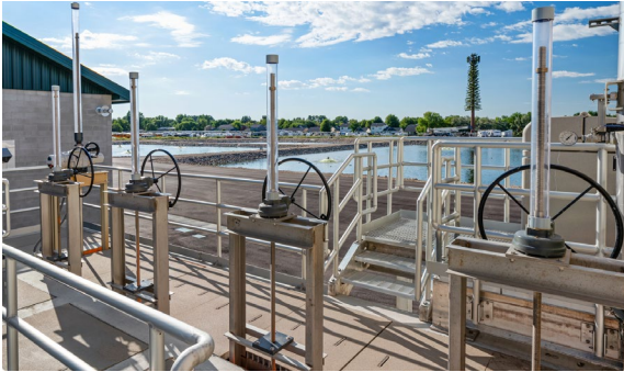
SSWD WWTP MBR Splitter Box
