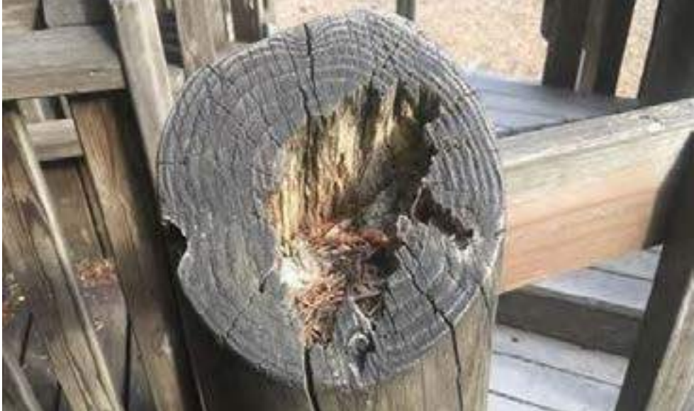
1. Splintering and declining wood frame
