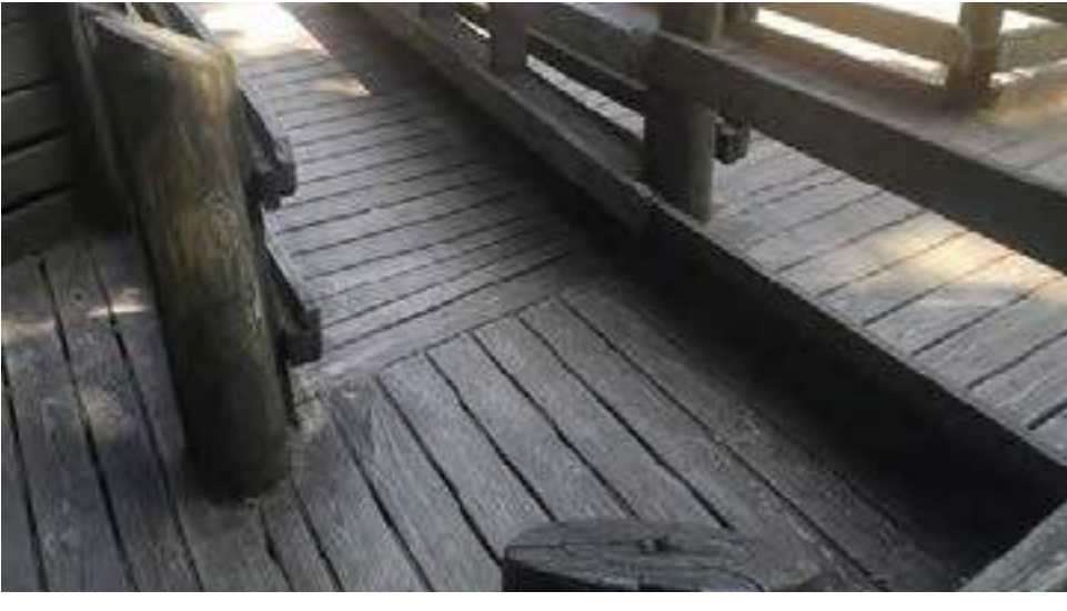
6. The current ADA accessible path is deteriorating, with visible signs of splitting and rot
