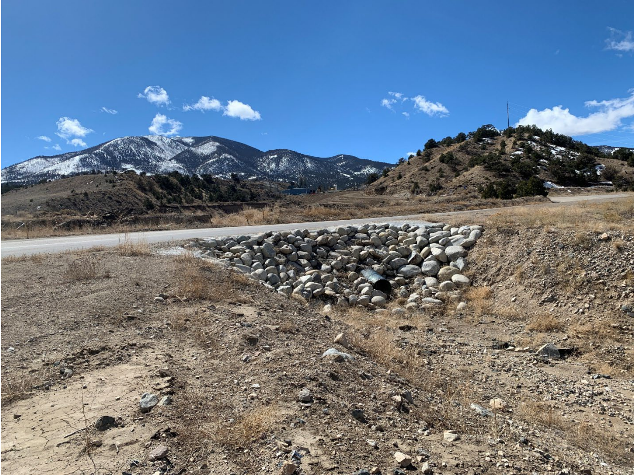
Runoff from basin 1 may split along CR107 and contribute to basin 2. This potential is due to the undersized culvert in the historic flow path at CR107, shown above. The undersized culvert should be addressed to prevent runoff from following CR107 from basin 1 into basin 2.
