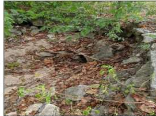
Half buried culvert at Rollingwood Drive. 09/11/2019
