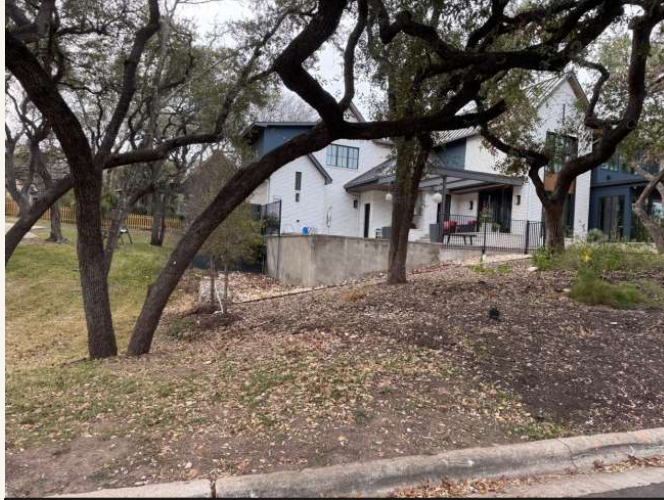
View from left corner of property - retaining wall visible from street level
