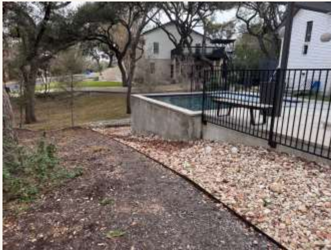
City-required riprap & French drain — occupies build-line area
