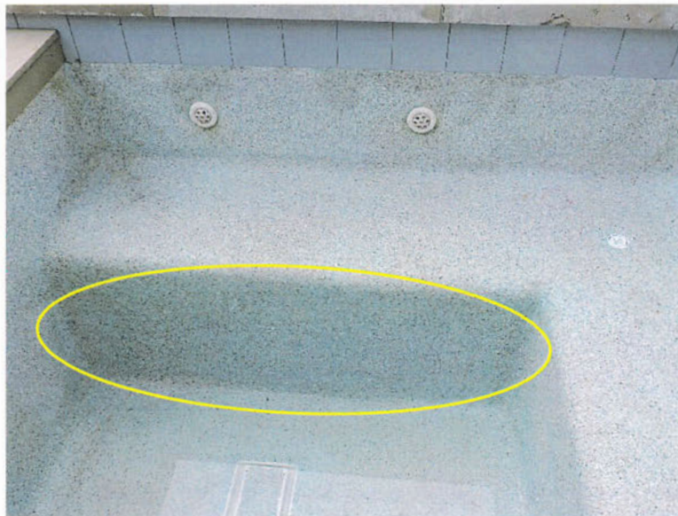
Figure 6: Cracking distress and efflorescence along bench of spa
