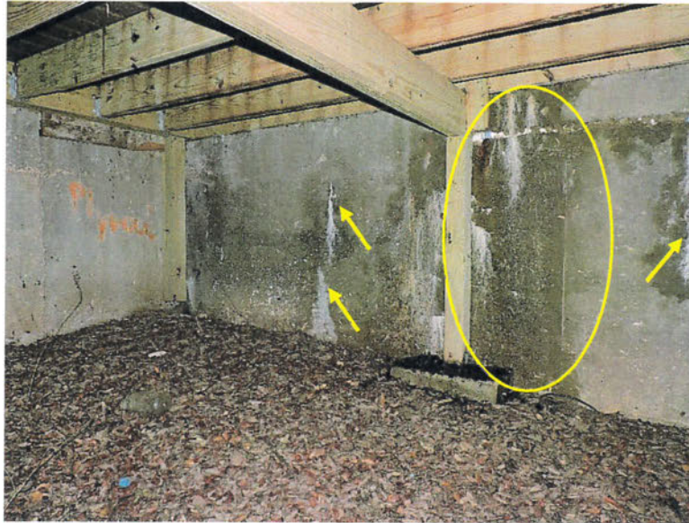
Figure 3: Cracking distress and efflorescence in crawl space underneath the pool deck
