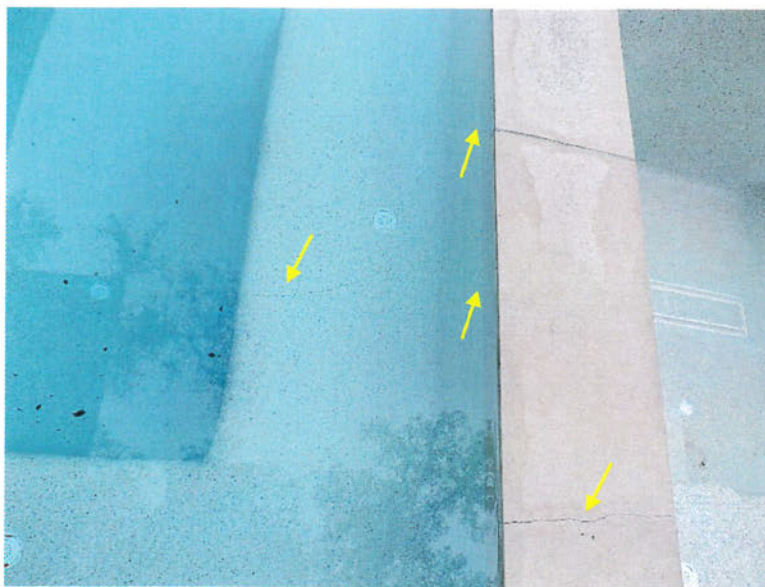
Figure 2: Cracking distress in bench along pool perimeter
