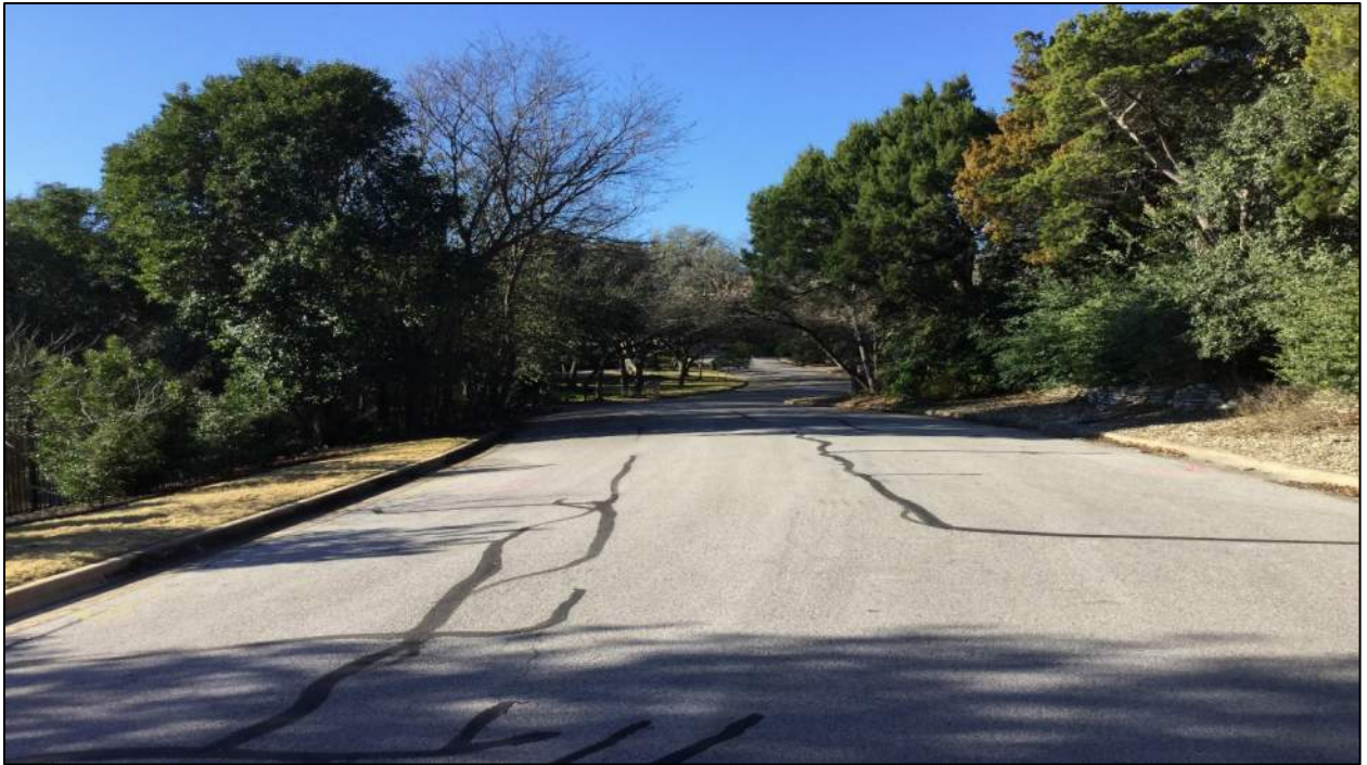
Photo 4: Viewing northwest on Pleasant Drive on the eastern side of the Review Area.
