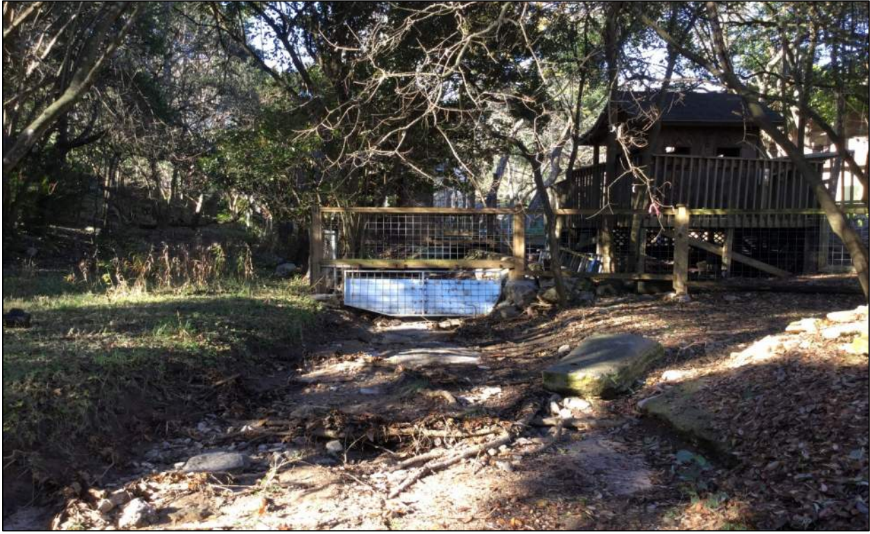
Photo 8: Viewing southwest in drainage channel behind 303 Nixon Drive on the eastern side of the Review Area.
